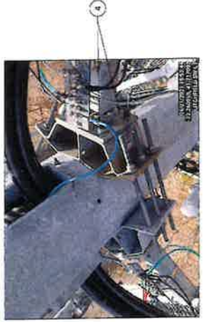
RUSTED BOLT AT MOUNT CONNECTION
