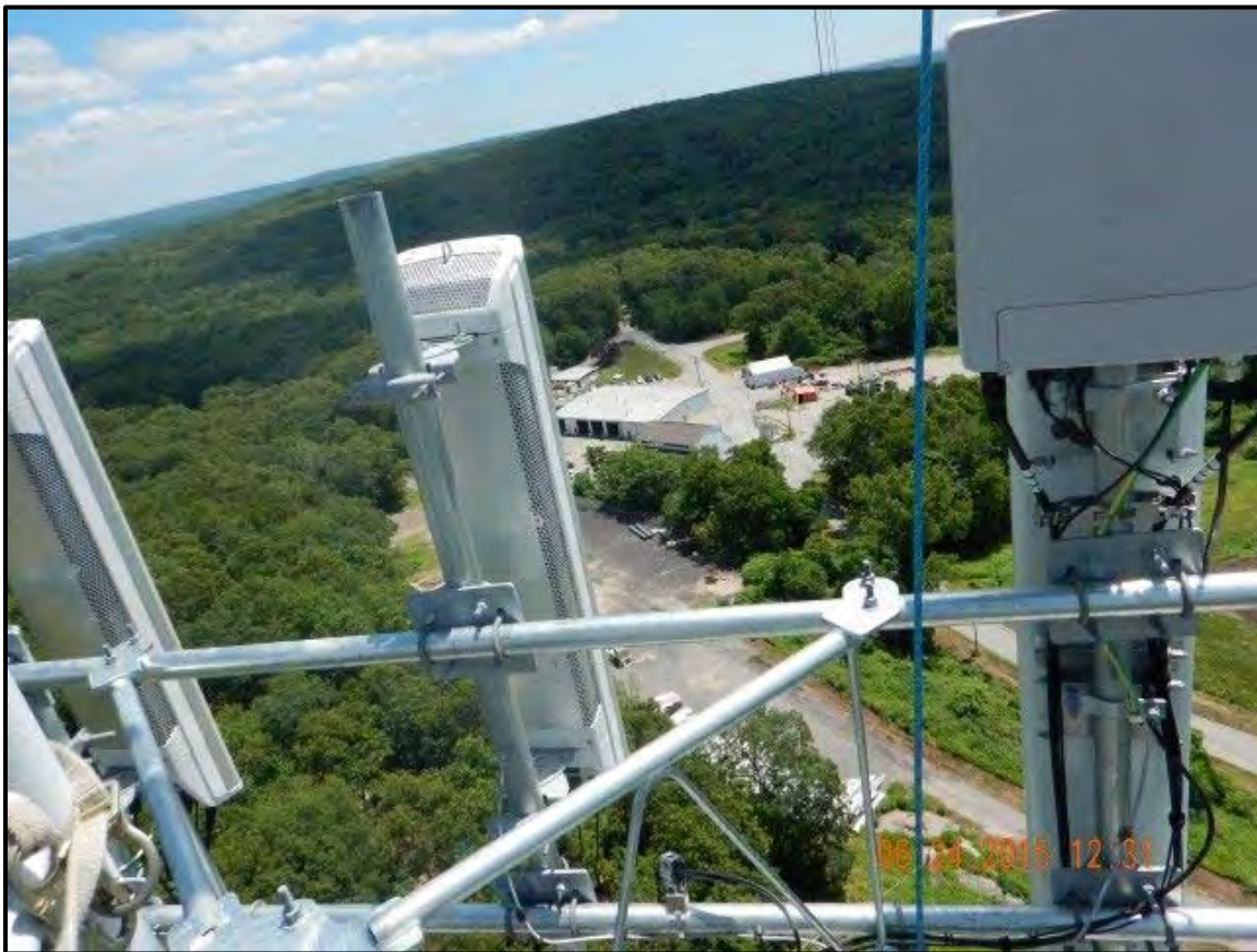
Existing T-Mobile Antenna Sector Mount on Tower
