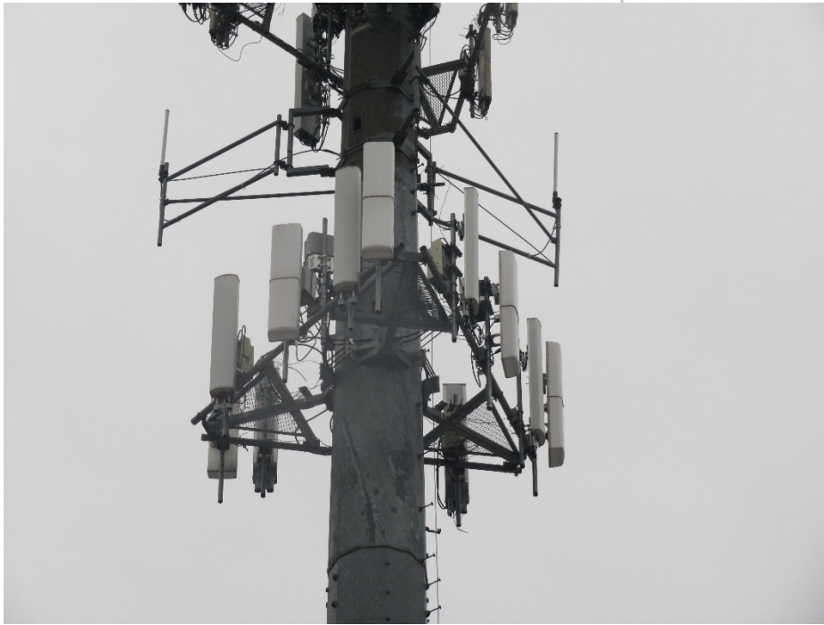
Photo 1: Photo illustrating the monopole with Appurtenances shown.
