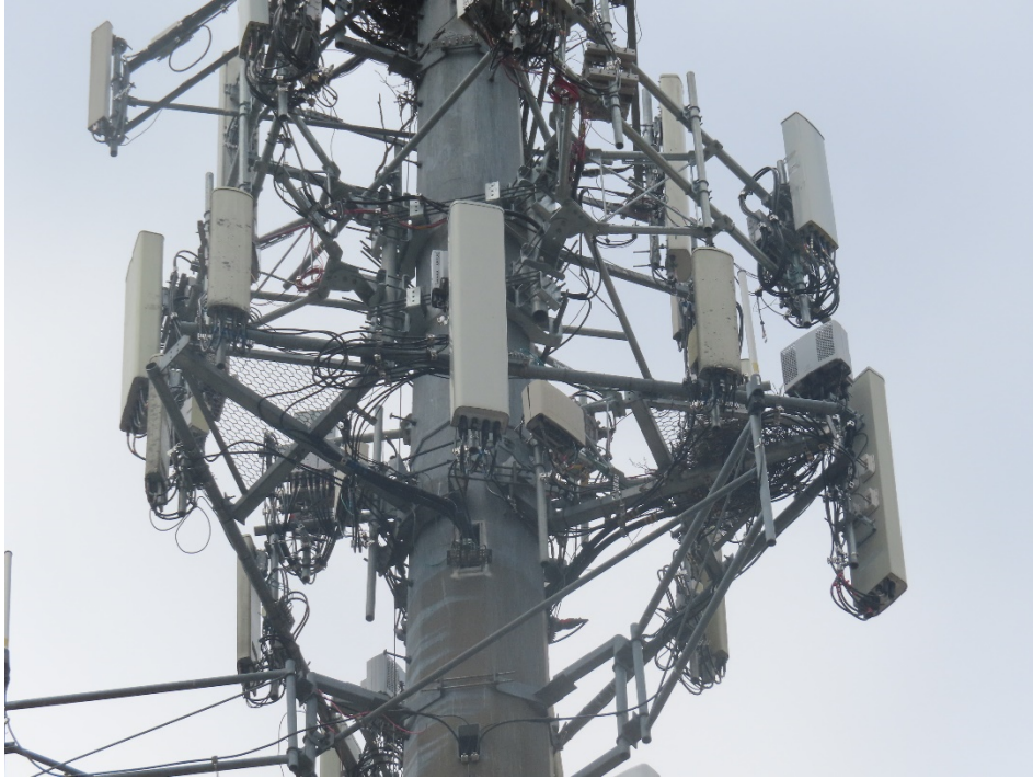
Photo 1: Photo illustrating the monopole with Appurtenances shown.
