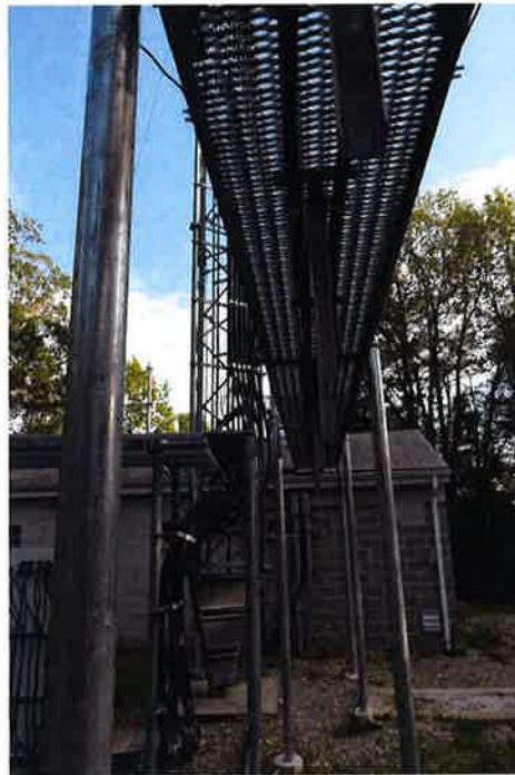
Photo of Verizon Wireless's ice bridge and feed lines.
