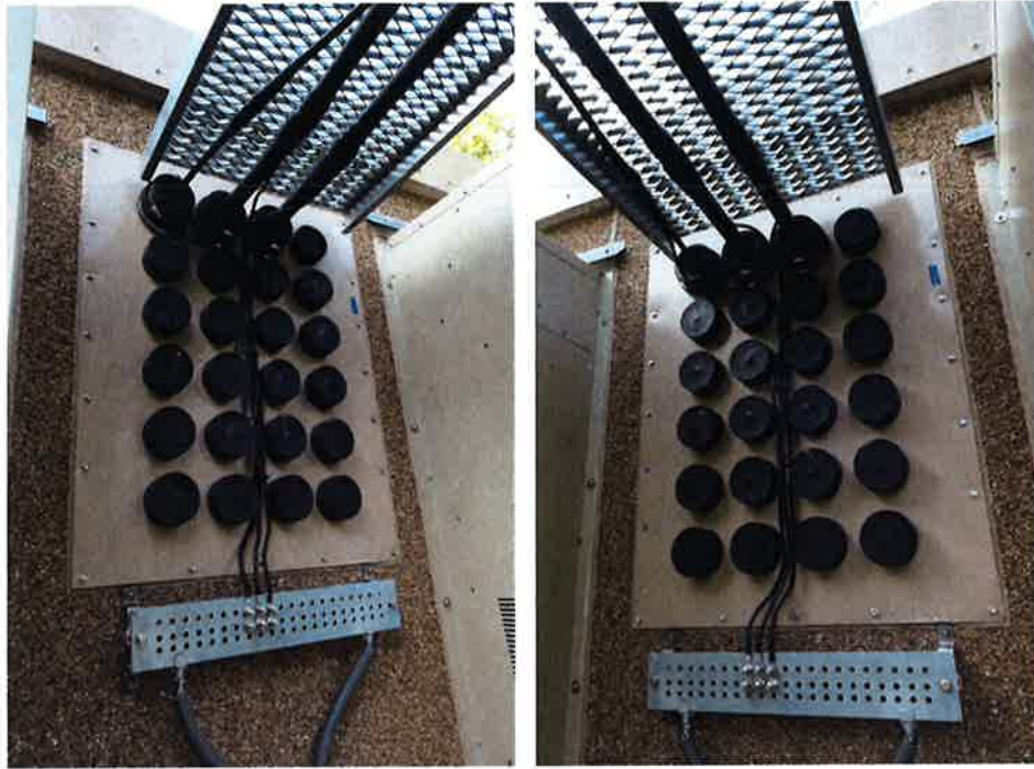
Photo of Verizon's existing feed lines at shelter.
