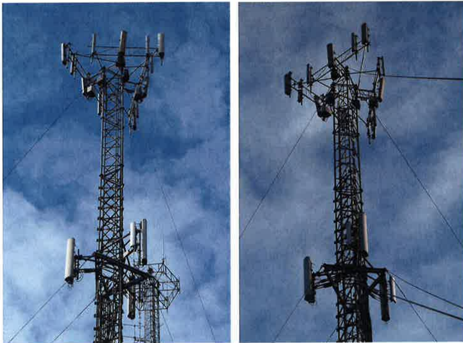
Photos of existing antennas. Verizon Wireless's equipment is top panel array.
