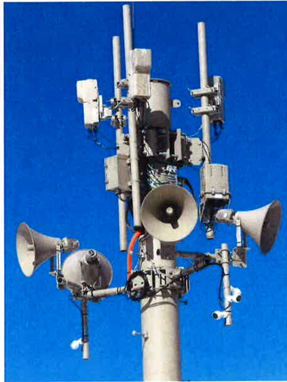
Image of existing Verizon and fairground pole mounted equipment.
