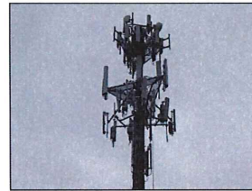
POSSIBLE MODIFICATION INTERFERENCE EL: 75'-0"± TO 87'-0"±
