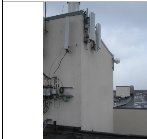
18. T-Mobile Sector B (Sprint B3 antenna to the left) roof view
