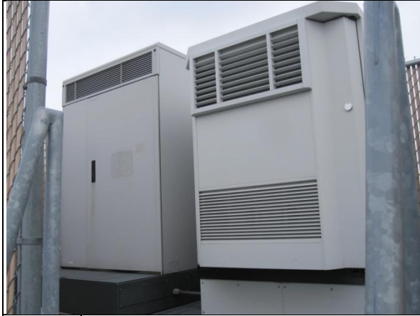
25. T-Mobile equipment cabinets
