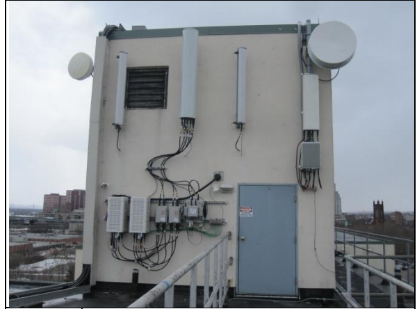
6. Sprint (3 left antennas) and Clearwire (right antenna) Sector A; microwave antennas to the left and right
