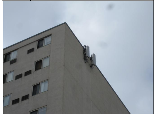
17. T-Mobile Sector A - ground view 2
