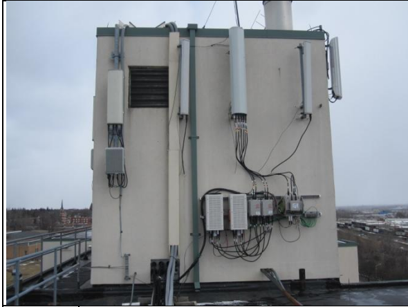
7. Sprint (3 right antennas) and Clearwire (left antenna) Sector B; T-Mobile Sector B to the right of Sprint
