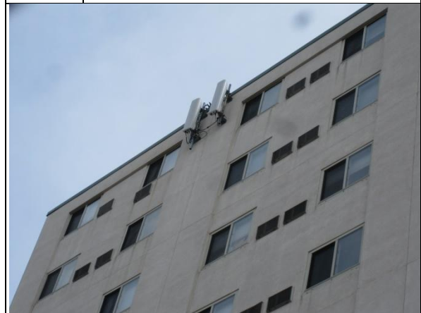
23. T-Mobile Sector C - ground view 2
