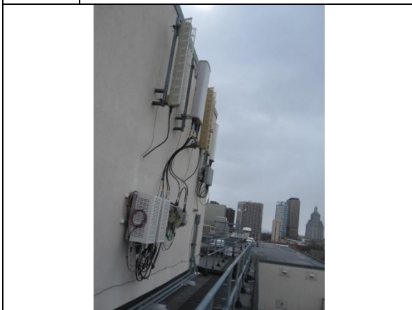
9. Sprint (3 left antennas) and Clearwire (right antenna) Sector C looking SW
