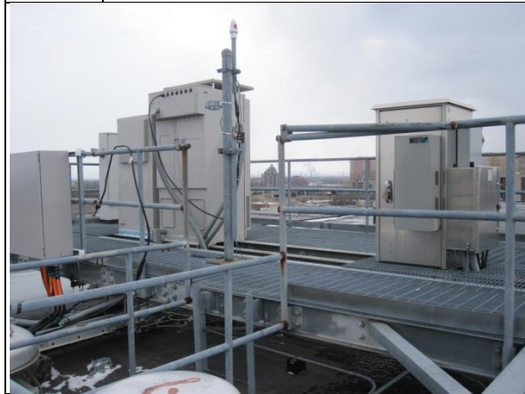
14. Sprint and Clearwire equipment
