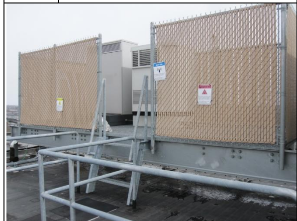
24. T-Mobile equipment compound
