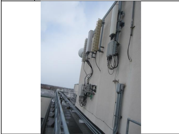
8. Sprint (3 left antennas) and Clearwire (right antenna) Sector C looking NE
