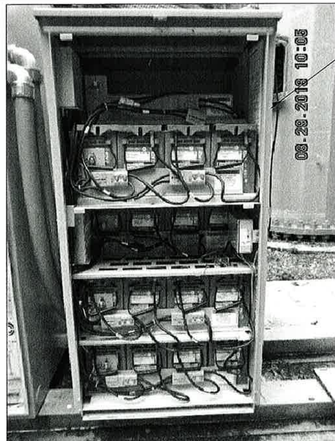
EXISTING BATTERY CABINET PHOTO
