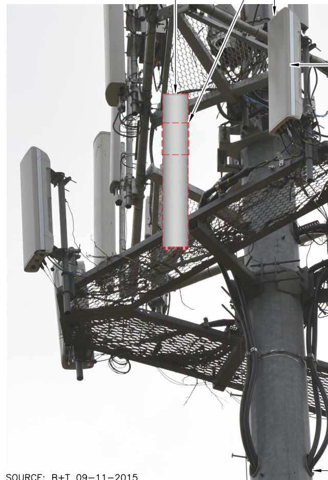
2 PROPOSED L700 T-MOBILE ANTENNA (1 PER SECTOR, TOTAL OF 3) (2/C-3) 1 PROPOSED RRU (1 PER SECTOR, TOTAL OF 3) (1/C-4) EXISTING T-MOBILE ANTENNAS AT 128'
