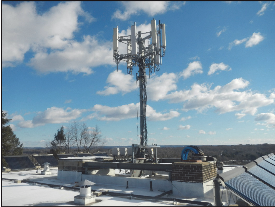
EXISTING MONOPOLE AND SUPPORTING STEEL PLATFORM ON ROOF
