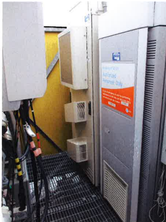
Photo 4: Sample photo illustrating the existing equipment cabinets.
