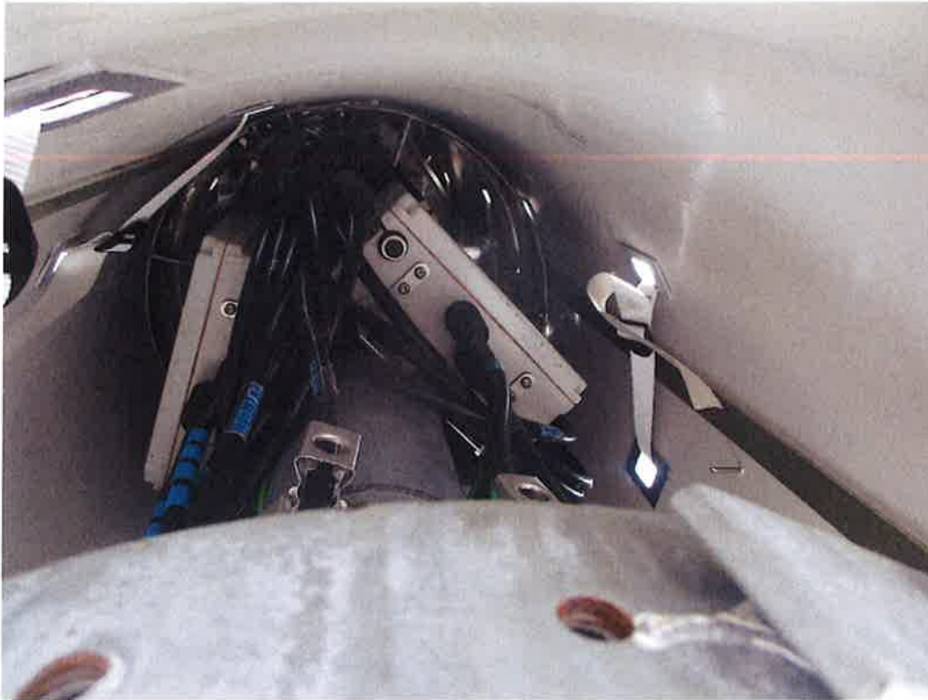
Photo 3: Sample photo illustrating the existing antennas and TMA's.
