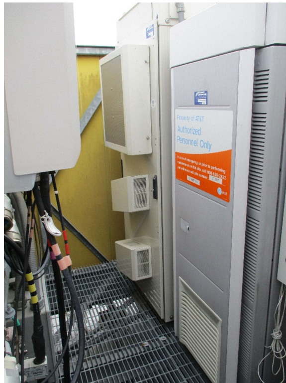
Photo 4: Sample photo illustrating the existing equipment cabinets.
