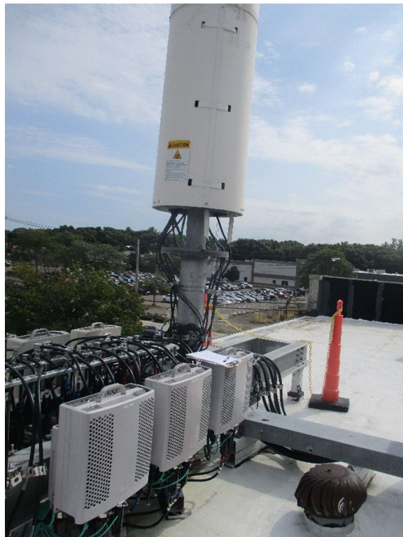
Photo 2: Sample photo illustrating the existing RRH's.
