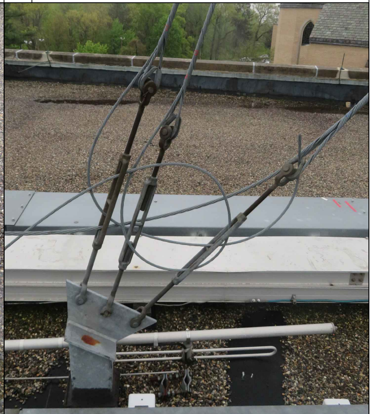
4. GUY ANCHOR AND WIRES
