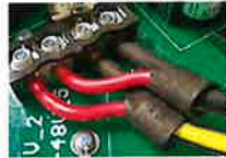
DC Wire Insulator
