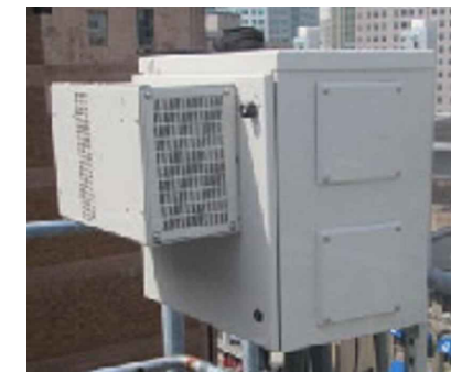
EMERSON NETXTEND COMPACT 2416 CABINET
