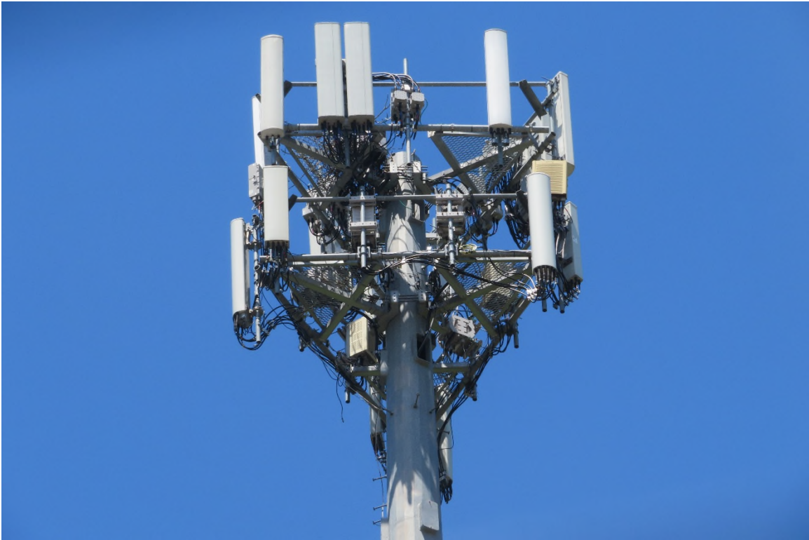
Photo 1: Photo illustrating the Tower with Appurtenances shown.
