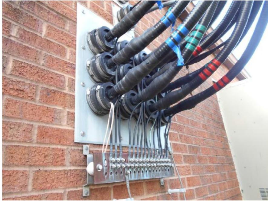
Photo of Verizon's existing hatch plates and ground bar at shelter.
