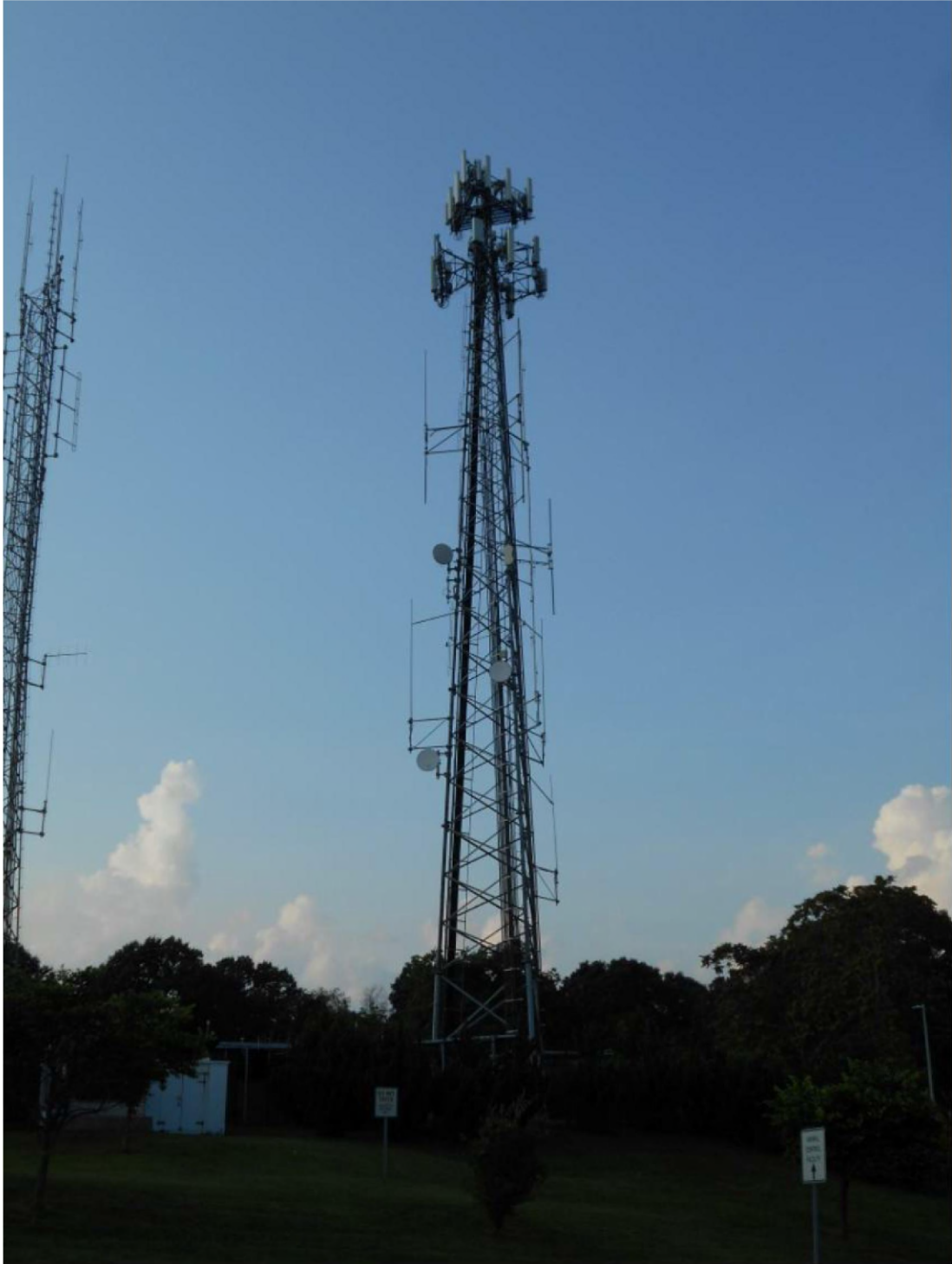
Overview photo of the existing 140' self-supporting tower structure located in Groton, Connecticut.
