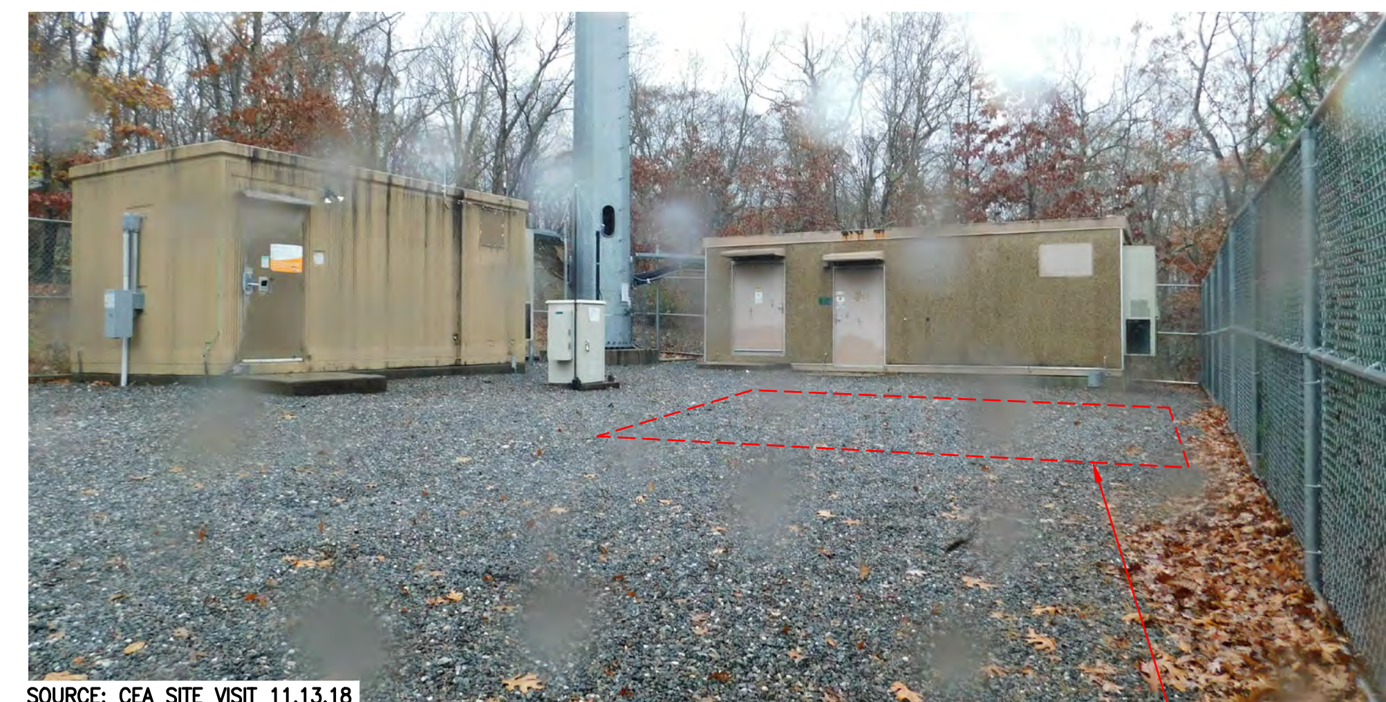
EQUIPMENT AREA PHOTO SCALE: N.T.S. 2 A-1 3 A-1 APPROX. LOCATION OF PROP. 10'x26' EQUIPMENT LEASE AREA
