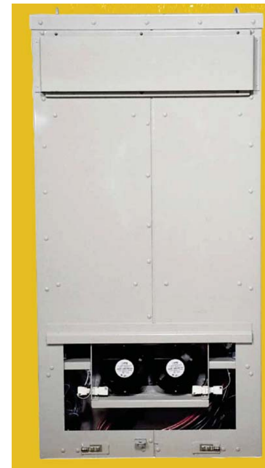
REAR VIEW GOECv2 BATTERY CABINET (REAR PANEL REMOVED)
