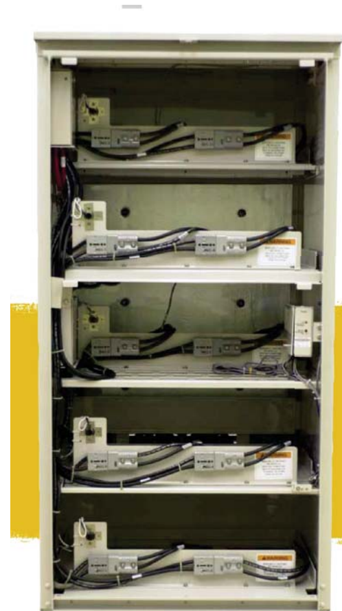
FRONT VIEW GOECv2 BATTERY CABINET (FRONT DOOR REMOVED)
