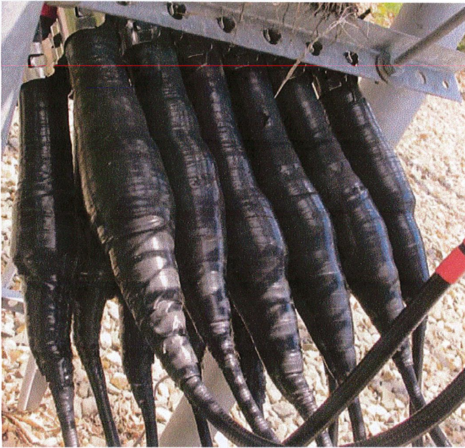
New & Existing coax cabling at equipment level.
