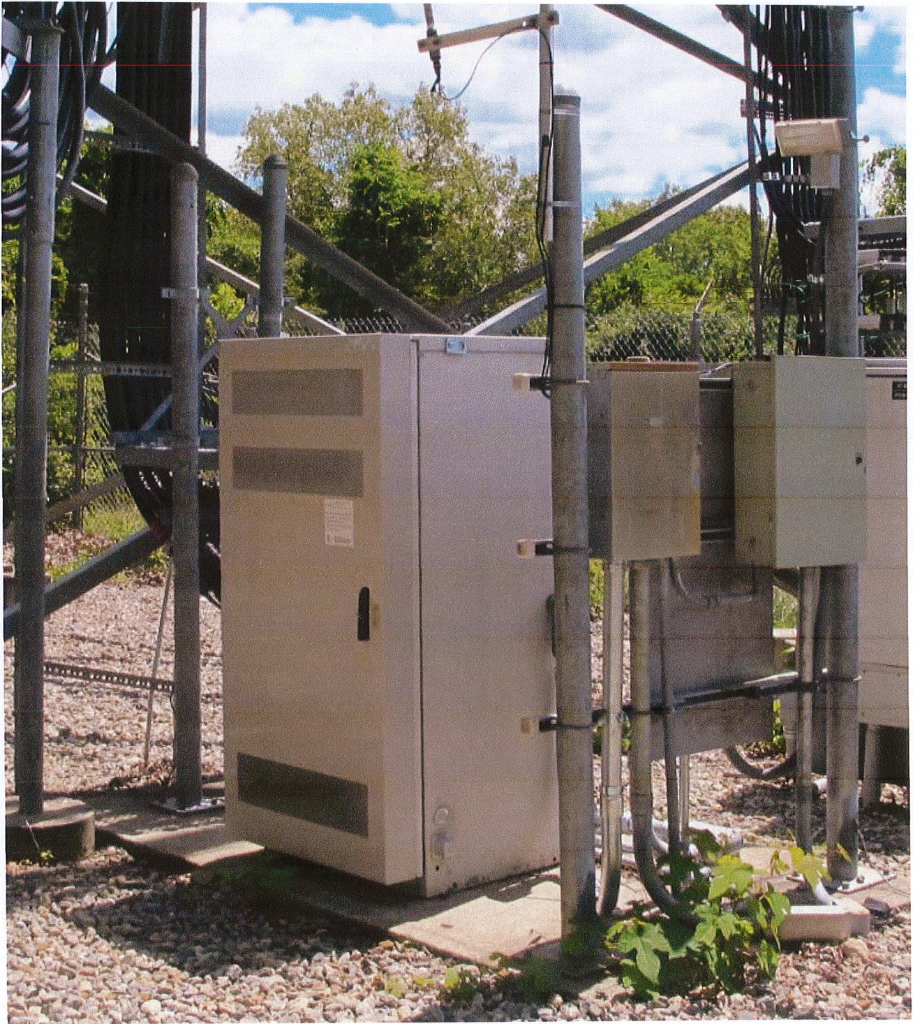
T-Mobile ground level equipment area.
