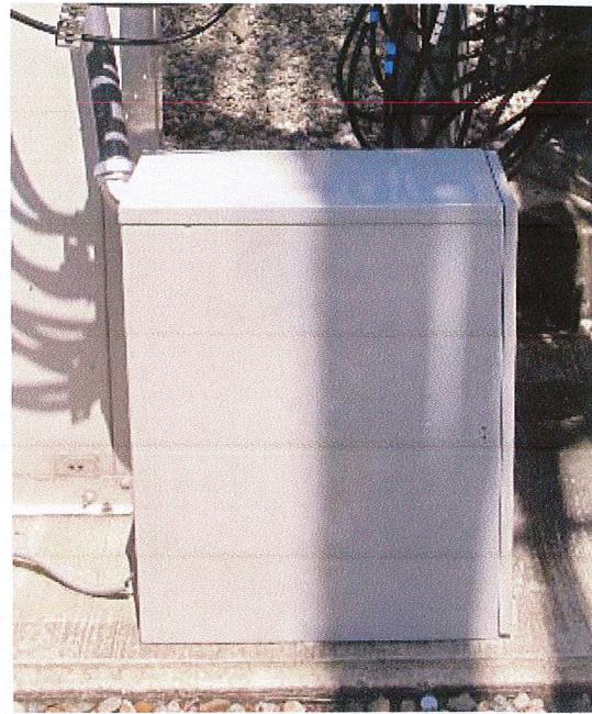
New Battery Backup Unit at equipment level.
