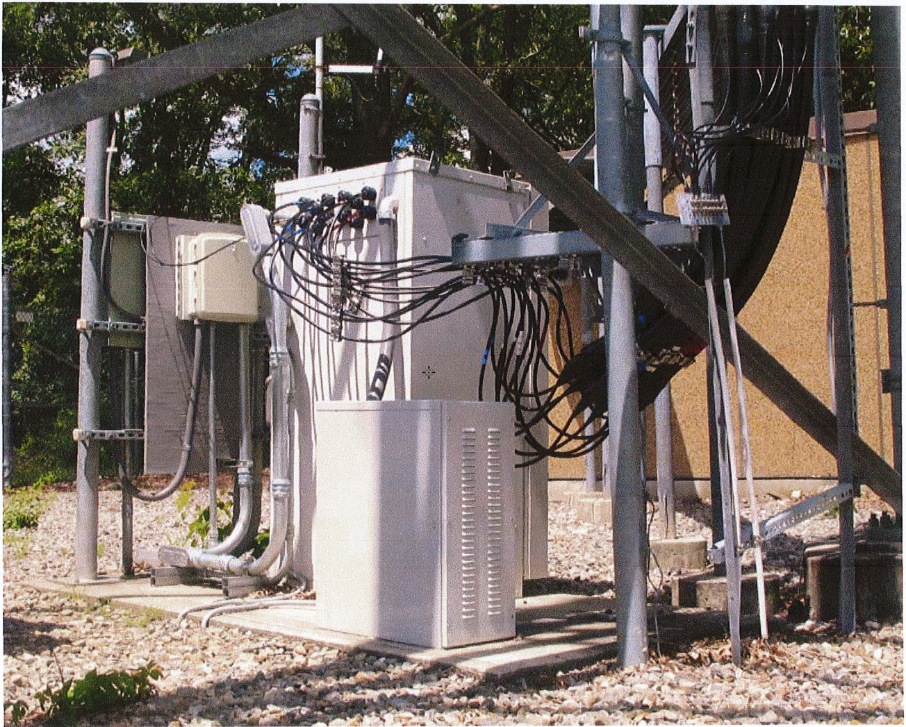
T-Mobile ground level equipment area.
