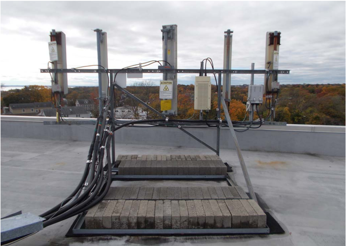
Existing Gamma Sector Ballast Frame
