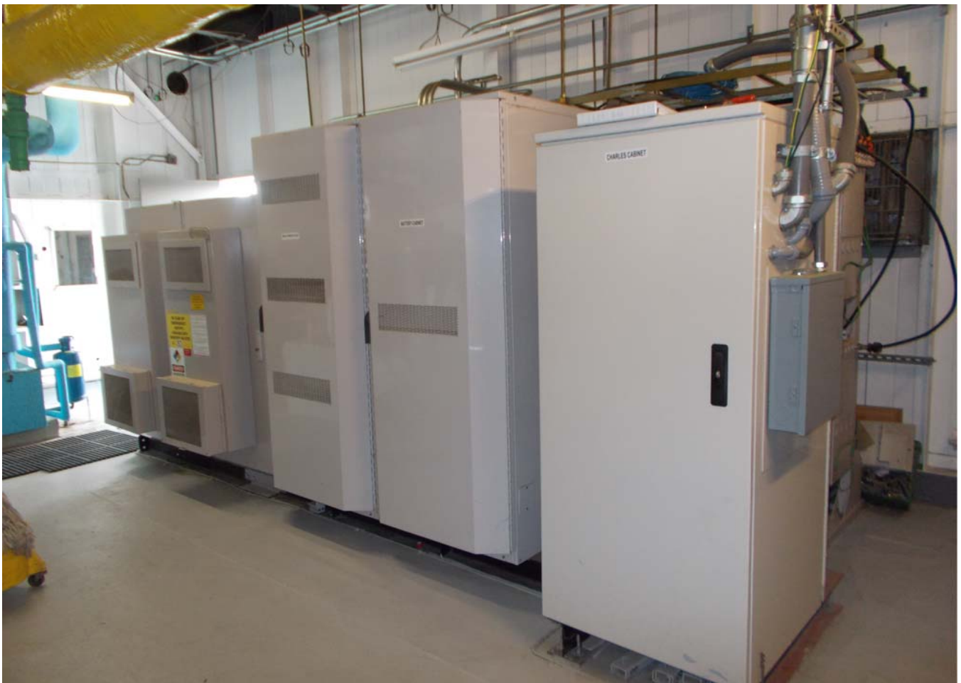
Existing Verizon Equipment in Penthouse Space
