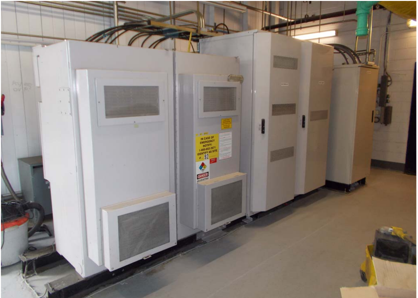
Existing Verizon Equipment in Penthouse Space
