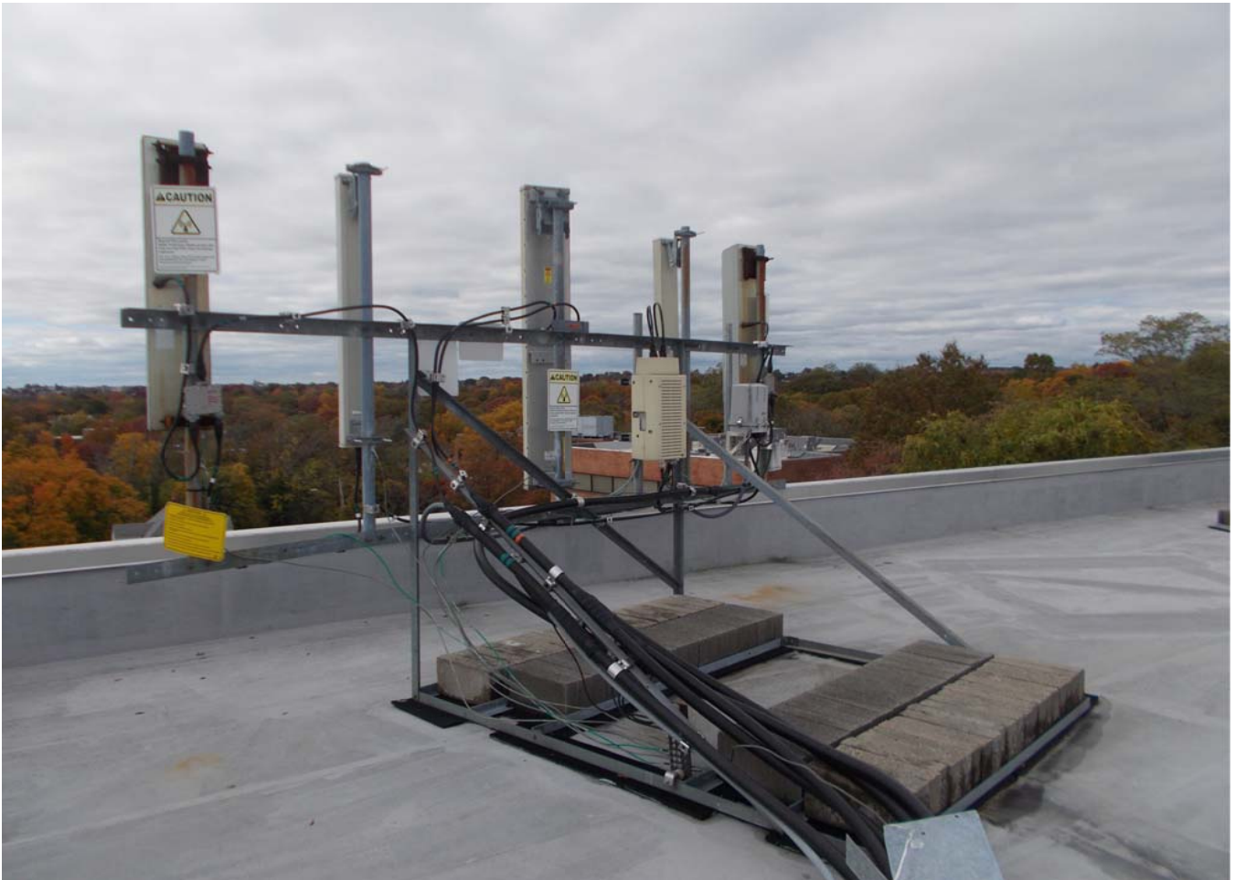
Existing Gamma Sector Ballast Frame
