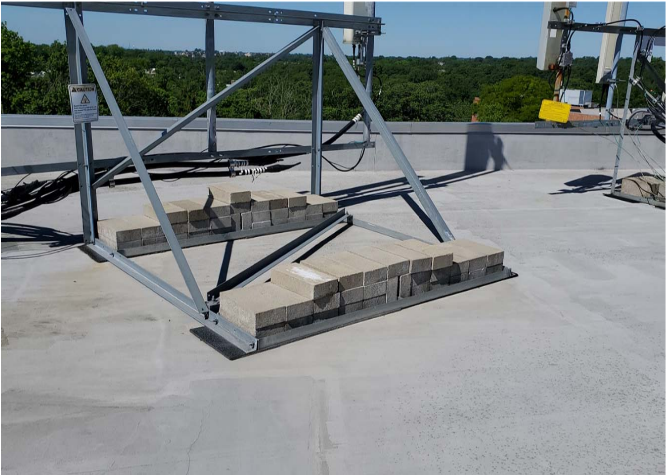
Existing T-Mobile Beta Sector Ballast
