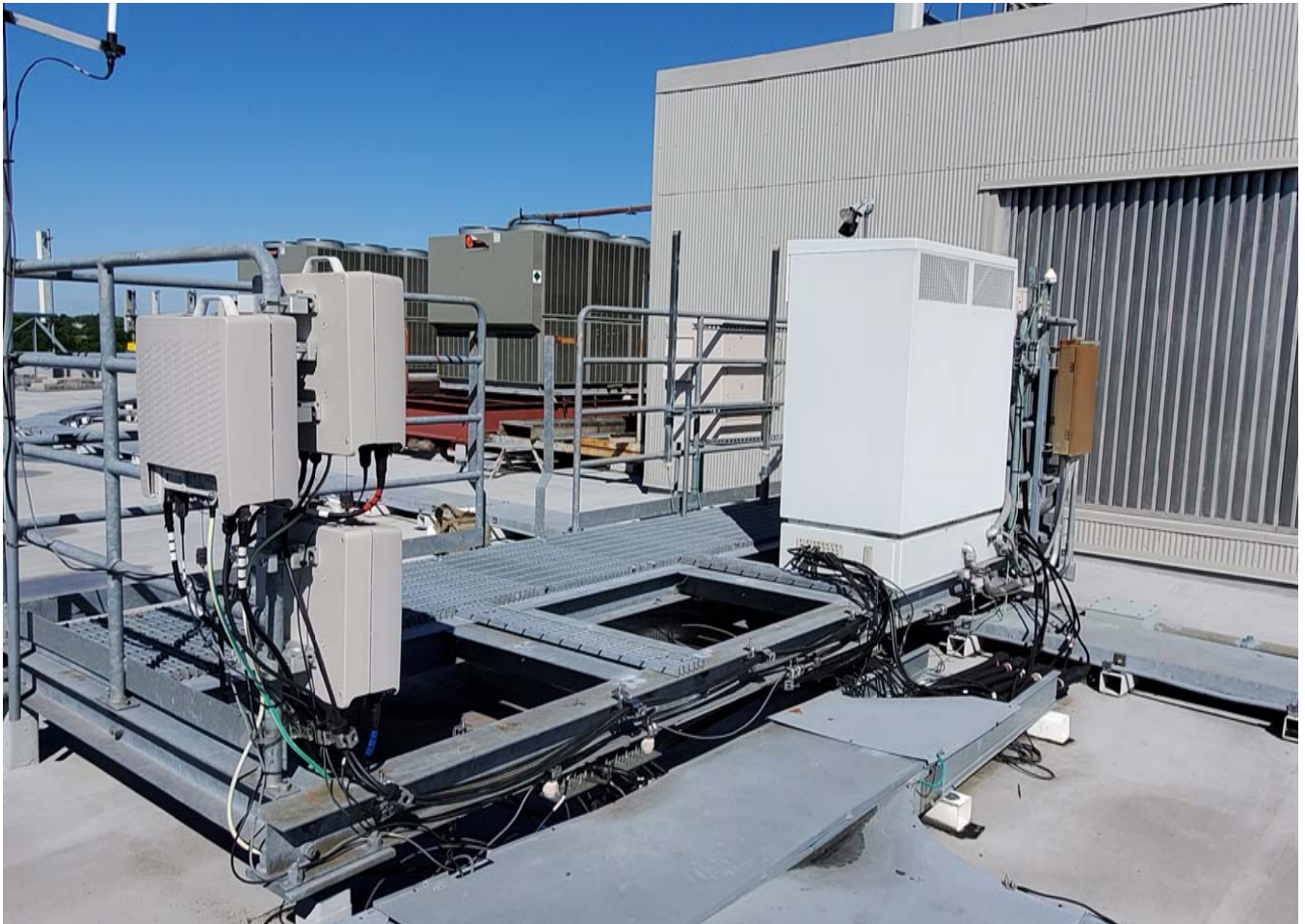
Existing T-Mobile Equipment Frame
