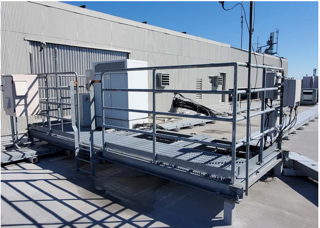
Existing T-Mobile Equipment Frame
