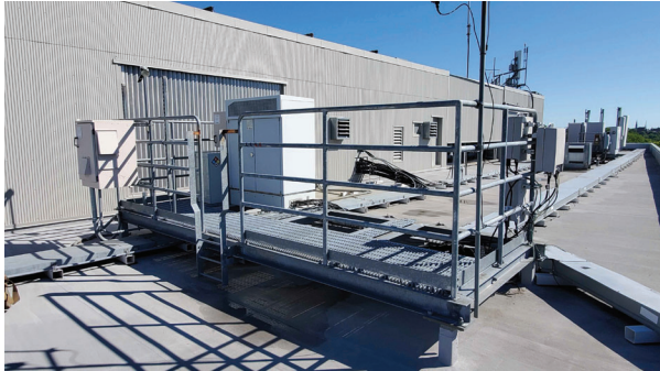
EXISTING EQUIPMENT PHOTO
