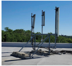
EXISTING BETA SECTOR ANTENNA PHOTO
