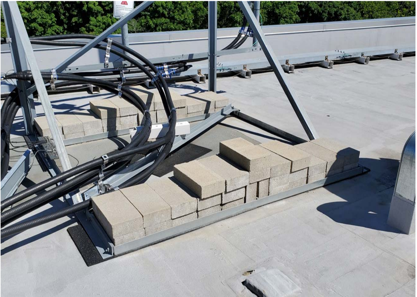
Existing T-Mobile Gamma Sector Ballast
