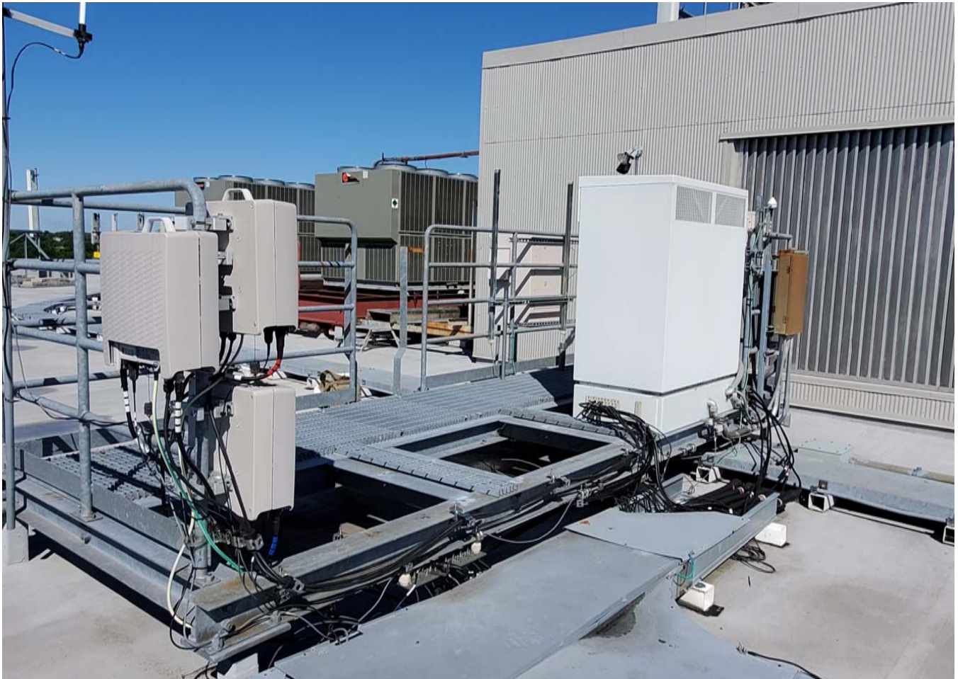
Existing T-Mobile Equipment Frame
