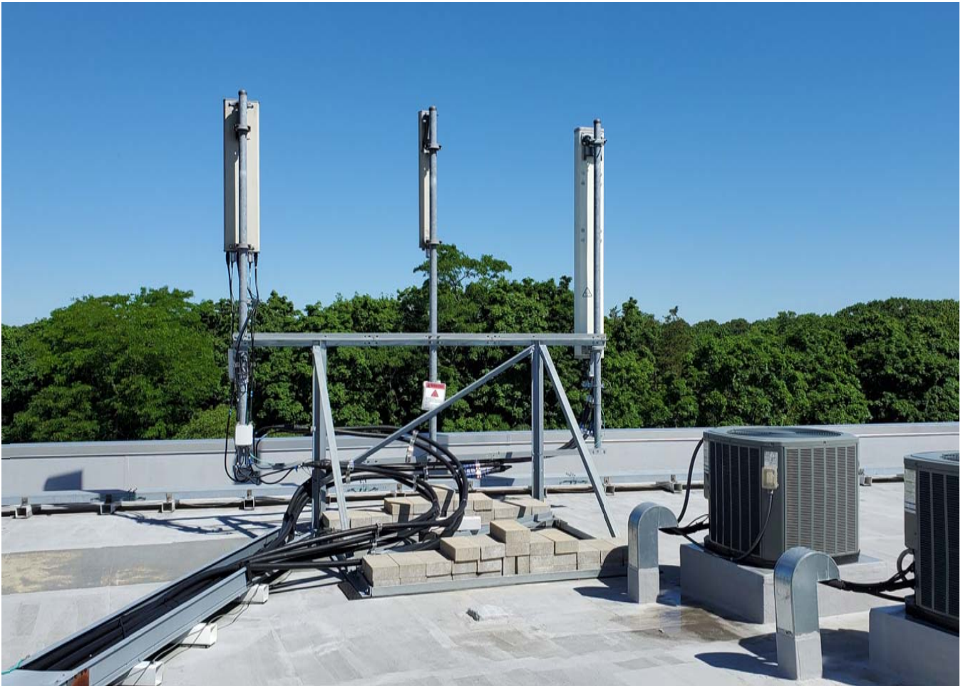
Existing T-Mobile Gamma Sector Antennas
