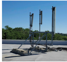
EXISTING BETA SECTOR ANTENNA PHOTO
