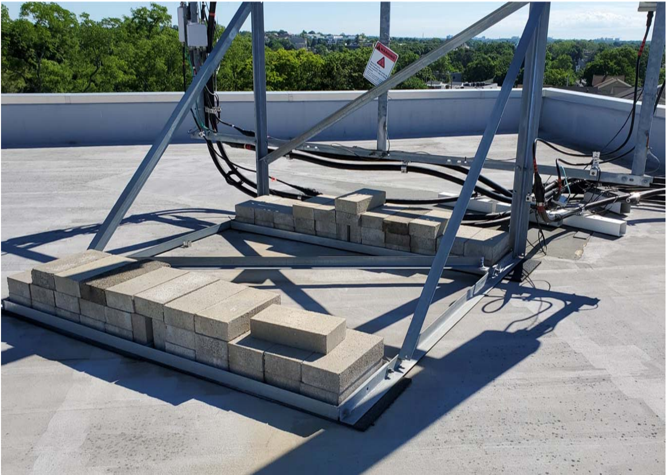
Existing T-Mobile Alpha Sector Ballast
