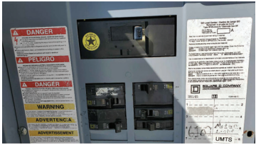
EXISTING POWER PANEL PHOTOS SCALE: NOT TO SCALE
