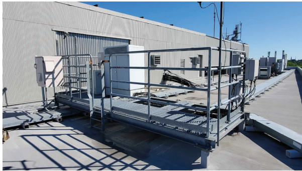
EXISTING EQUIPMENT PHOTO
