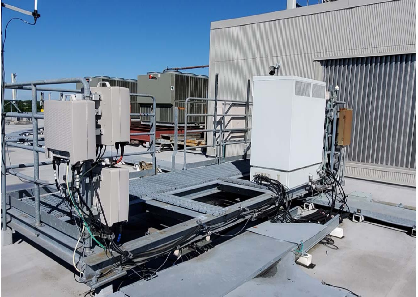
Existing T-Mobile Equipment Frame
