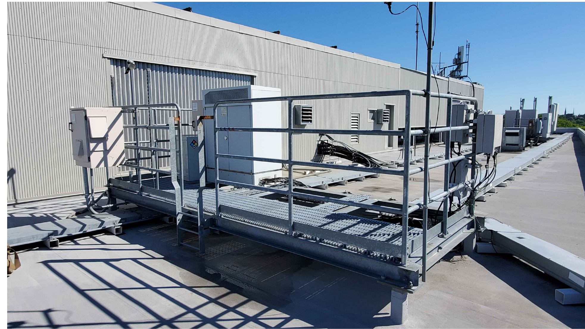
EXISTING EQUIPMENT PHOTO
