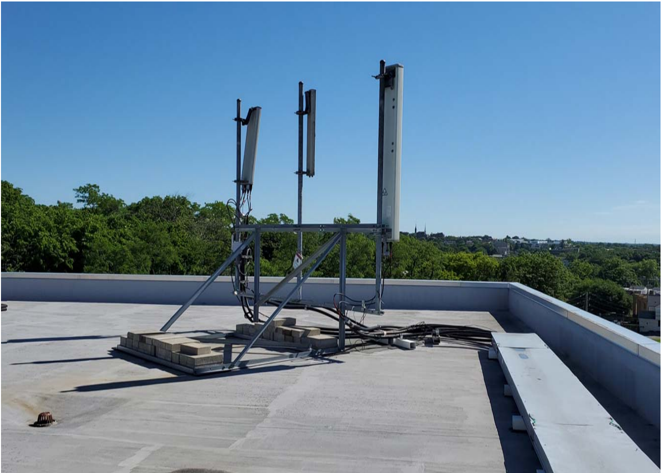
Existing T-Mobile Alpha Sector Antennas
