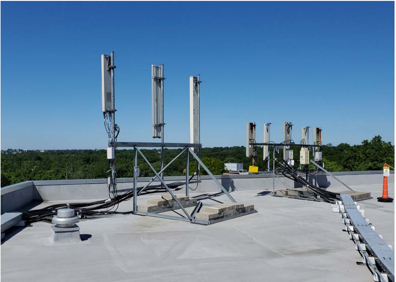
Existing T-Mobile Beta Sector Antennas
