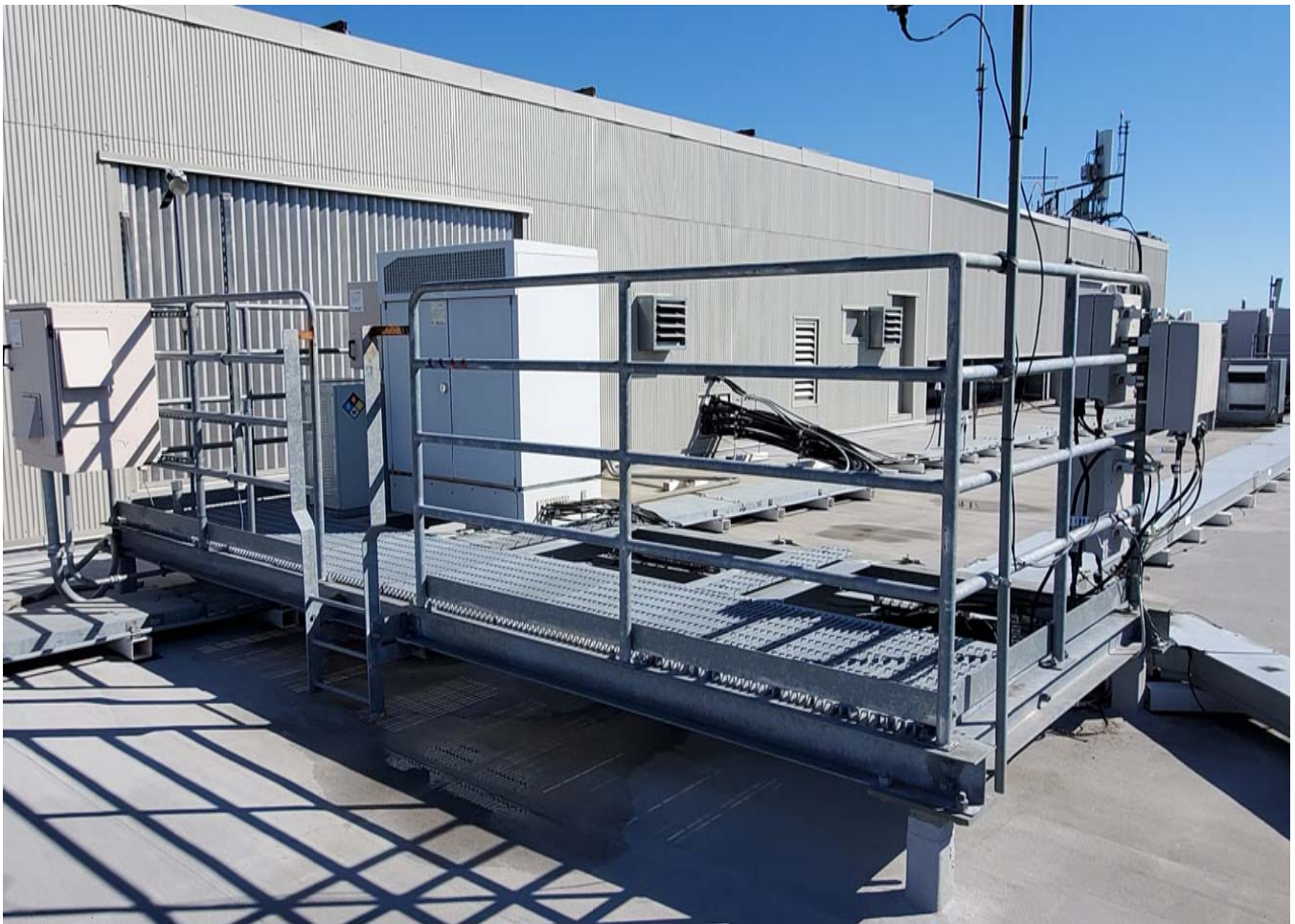
Existing T-Mobile Equipment Frame
