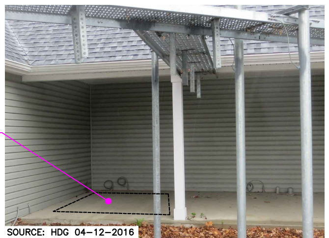
EQUIPMENT LOCATION PHOTO DETAIL SCALE: N.T.S. 3 A-1
