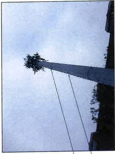
Existing Safety Cable
