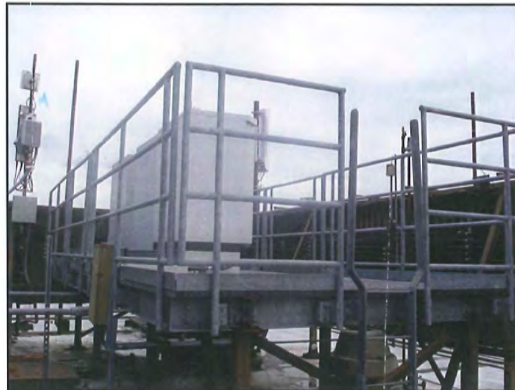
Existing equipment on the rooftop
