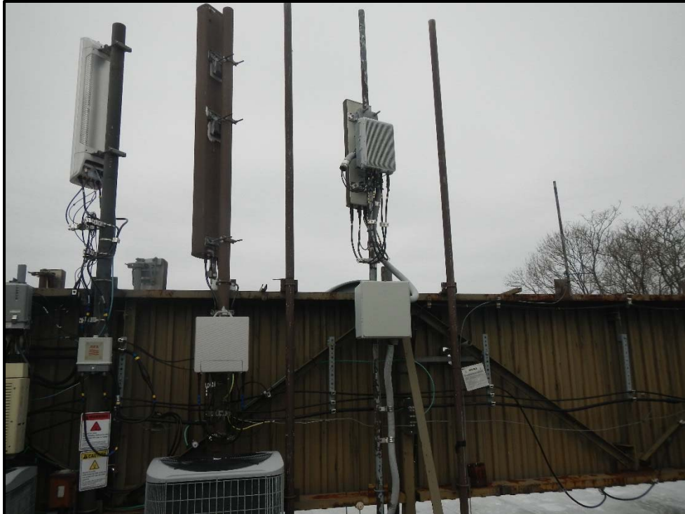
Existing Gamma Sector Pipe Mounts on Roof Screen
