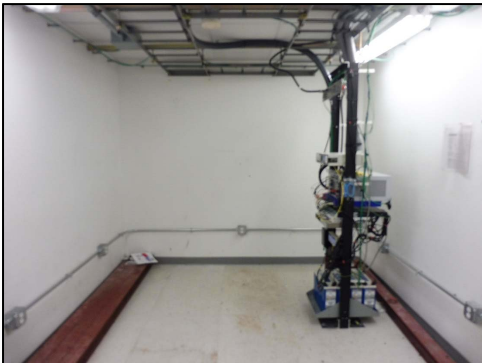
Overview of Equipment Room
