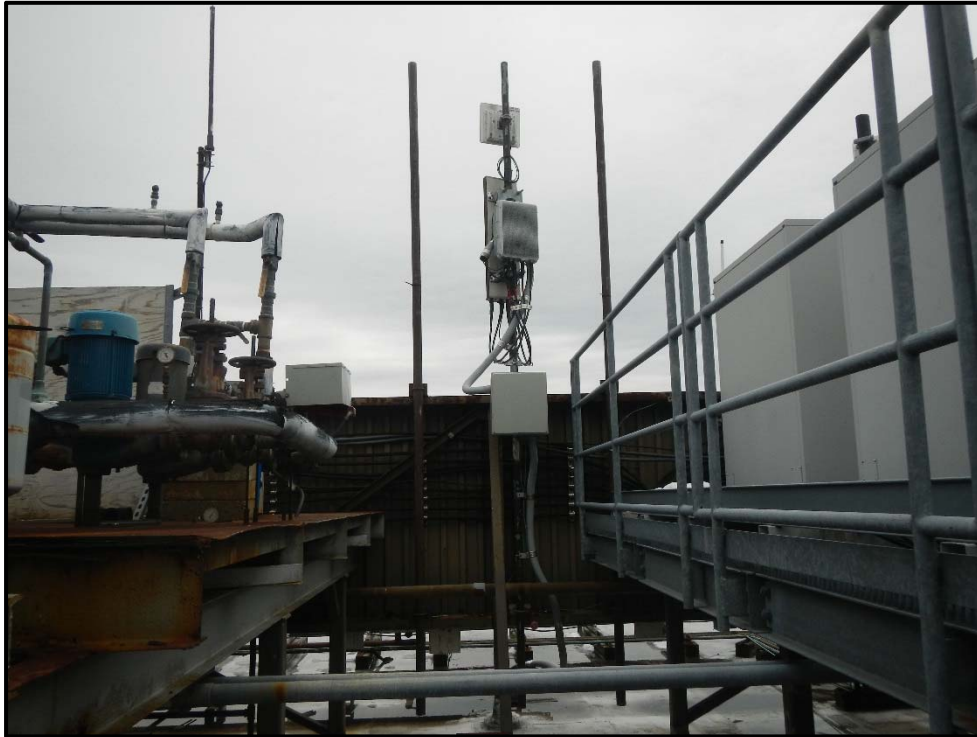
Existing Alpha Sector Pipe Mounts on Roof Screen
