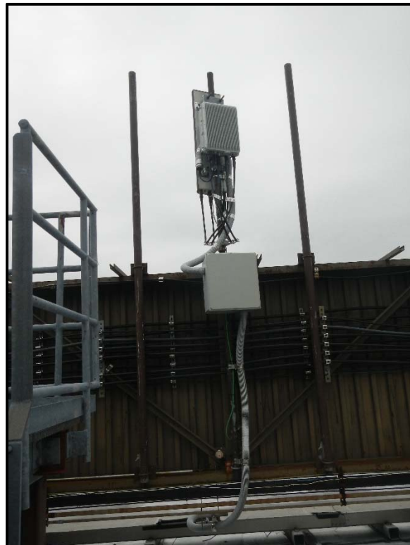
Existing Beta Sector Pipe Mounts on Roof Screen
