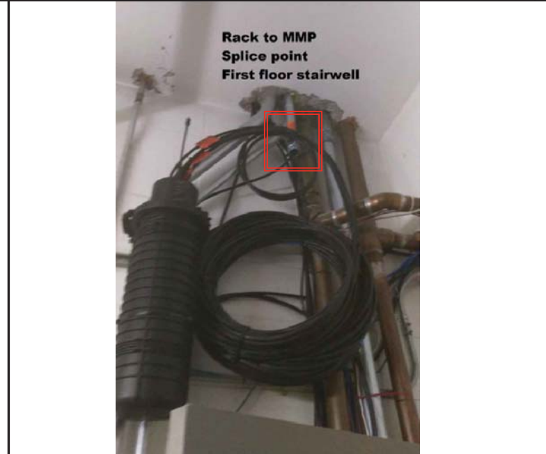
CONDUIT PENETRATION INTO FIRST FLOOR STAIRWELL
