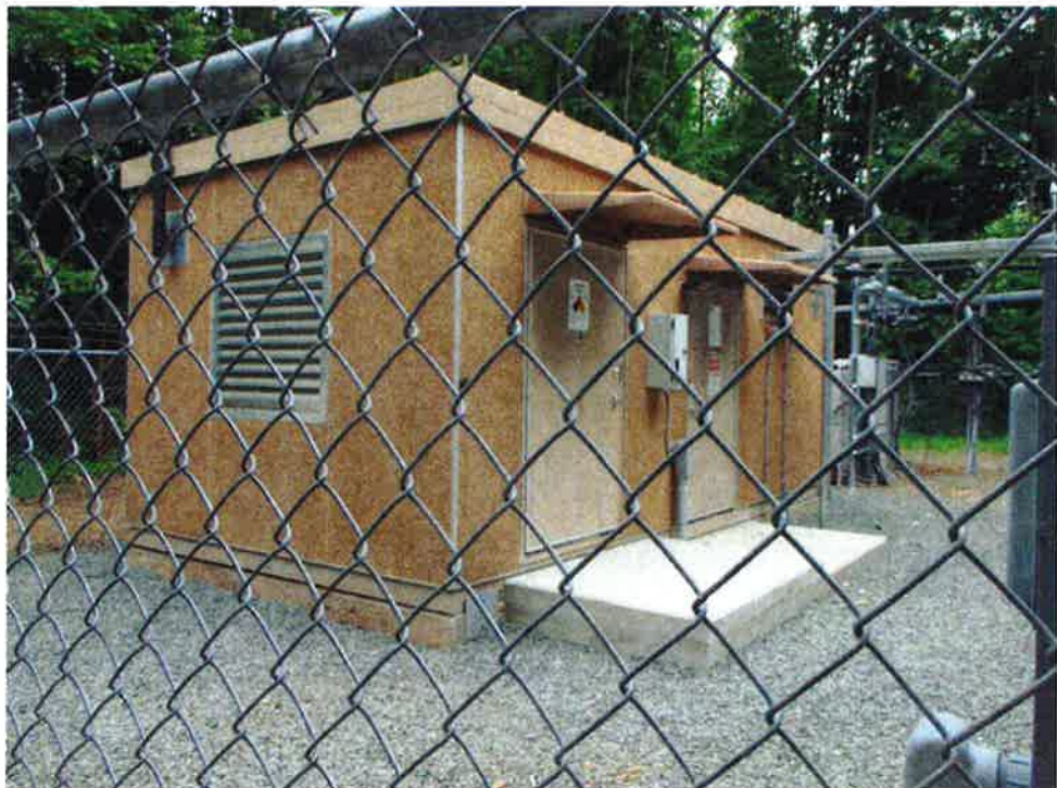
Figure 3: Verizon Equipment Shelter
