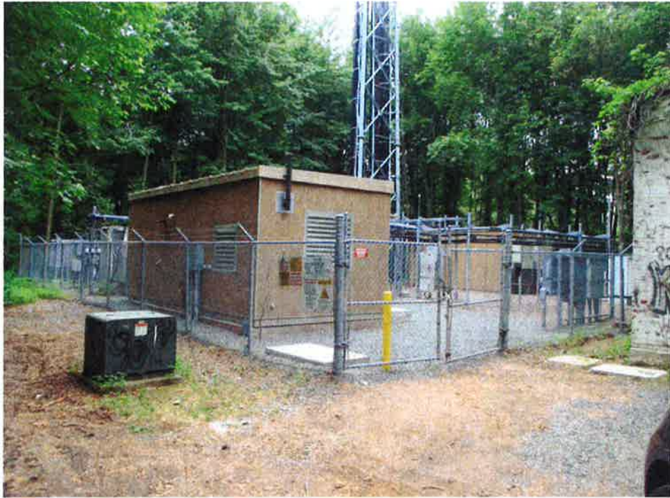
Figure 2: Fenced Equipment Compound
