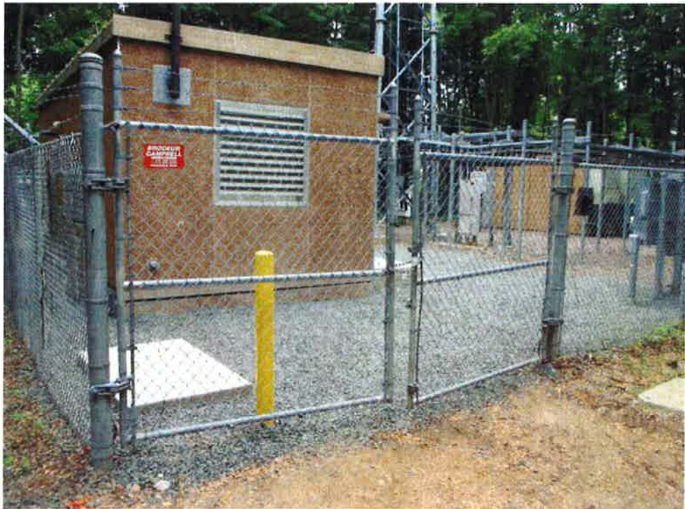
Figure 4: Equipment Compound Gate
