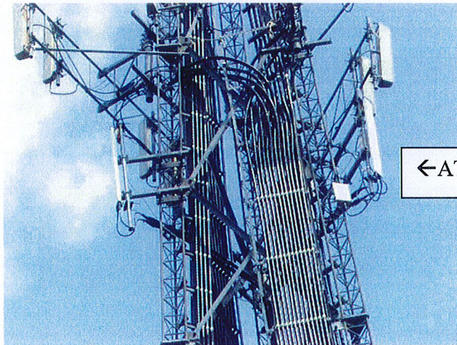
AT&T ARRAY TO BE REMOVED, SHOWN AT 152' LEVEL
