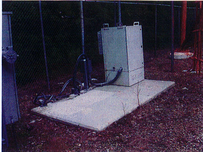
AT&T GROUND EQUIPMENT TO BE REMOVED
