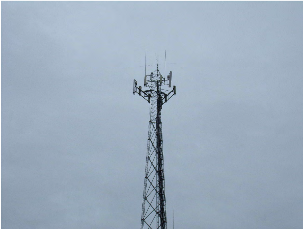
Photo 1: Photo illustrating the Tower with Appurtenances shown.
