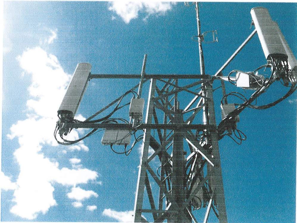
Photo 1: existing antennas mounted to the tower
