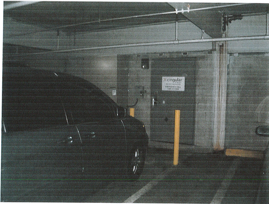
Photo 2: Existing equipment room in the parking garage below the building
