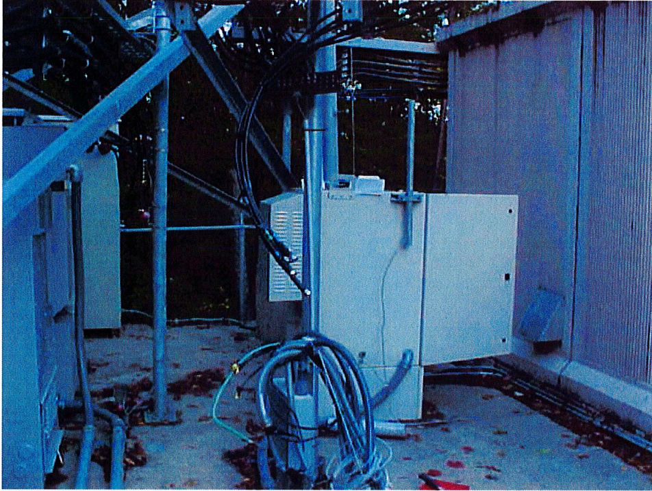
AT&T Base station and equipment before removal
