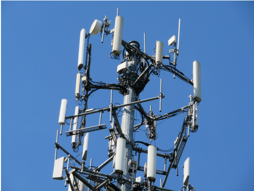
Photo 1: Photo illustrating the Monopole with Appurtenances shown.
