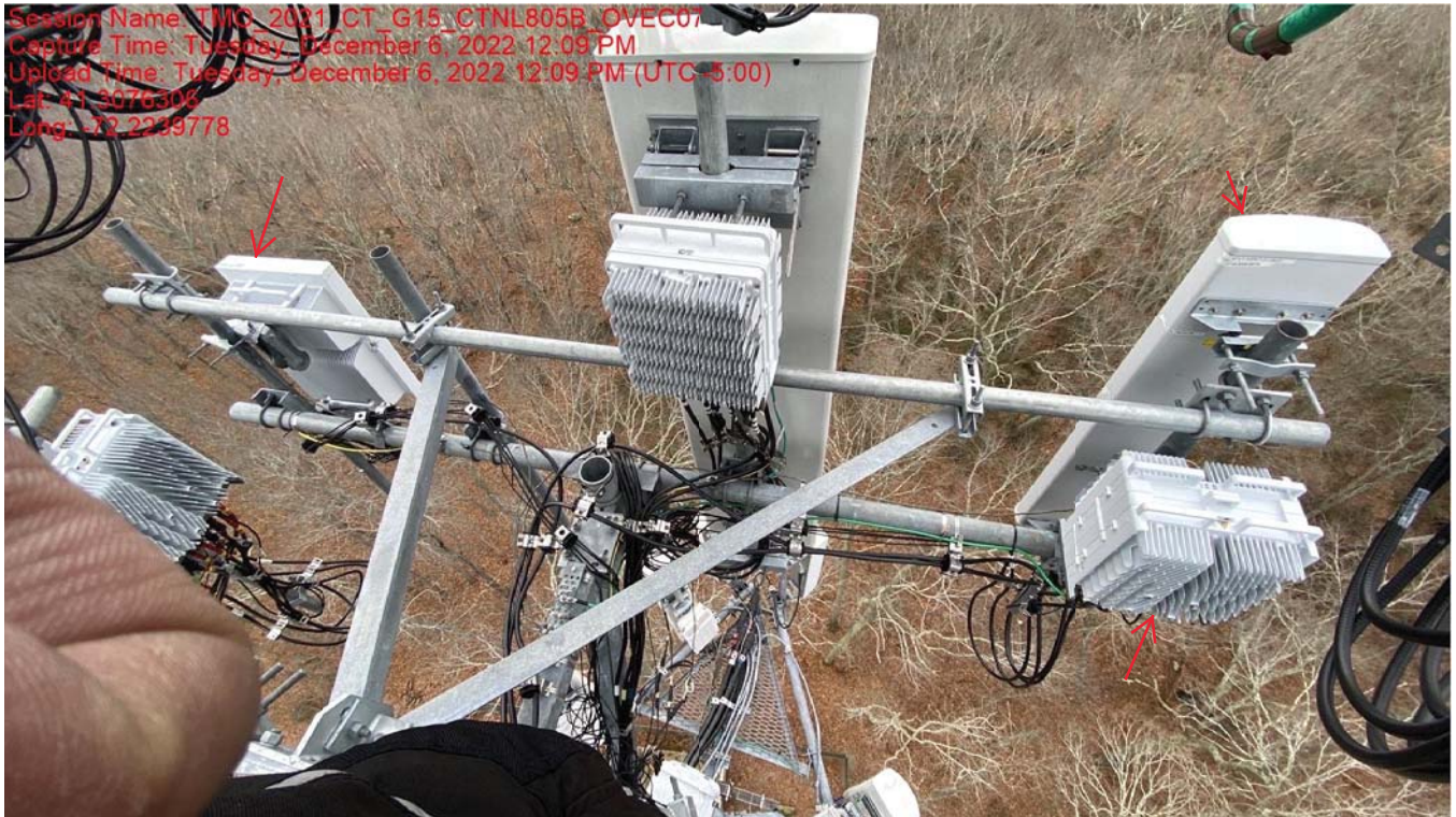
Beta Sector: (2) New Antennas & (1) New RRH Mounted To Existing Sector Frame
