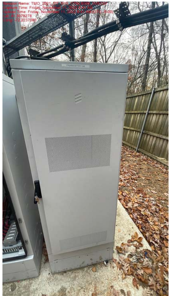
New Battery Cabinet Mounted To Concrete Pad
