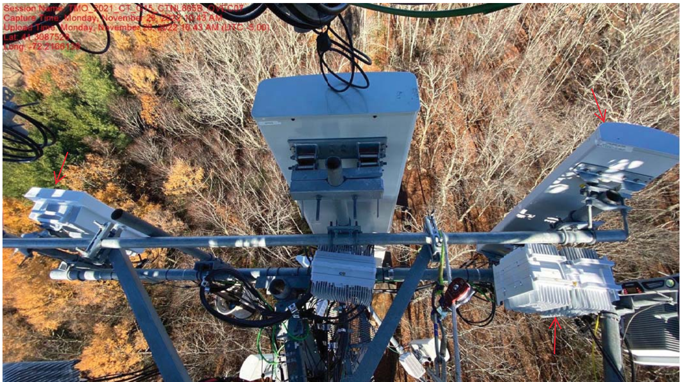
Alpha Sector: (2) New Antennas & (1) New RRH Mounted To Existing Sector Frame
