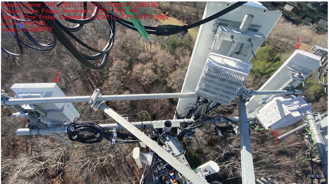
Gamma Sector: (2) New Antennas & (1) New RRH Mounted To Existing Sector Frame
