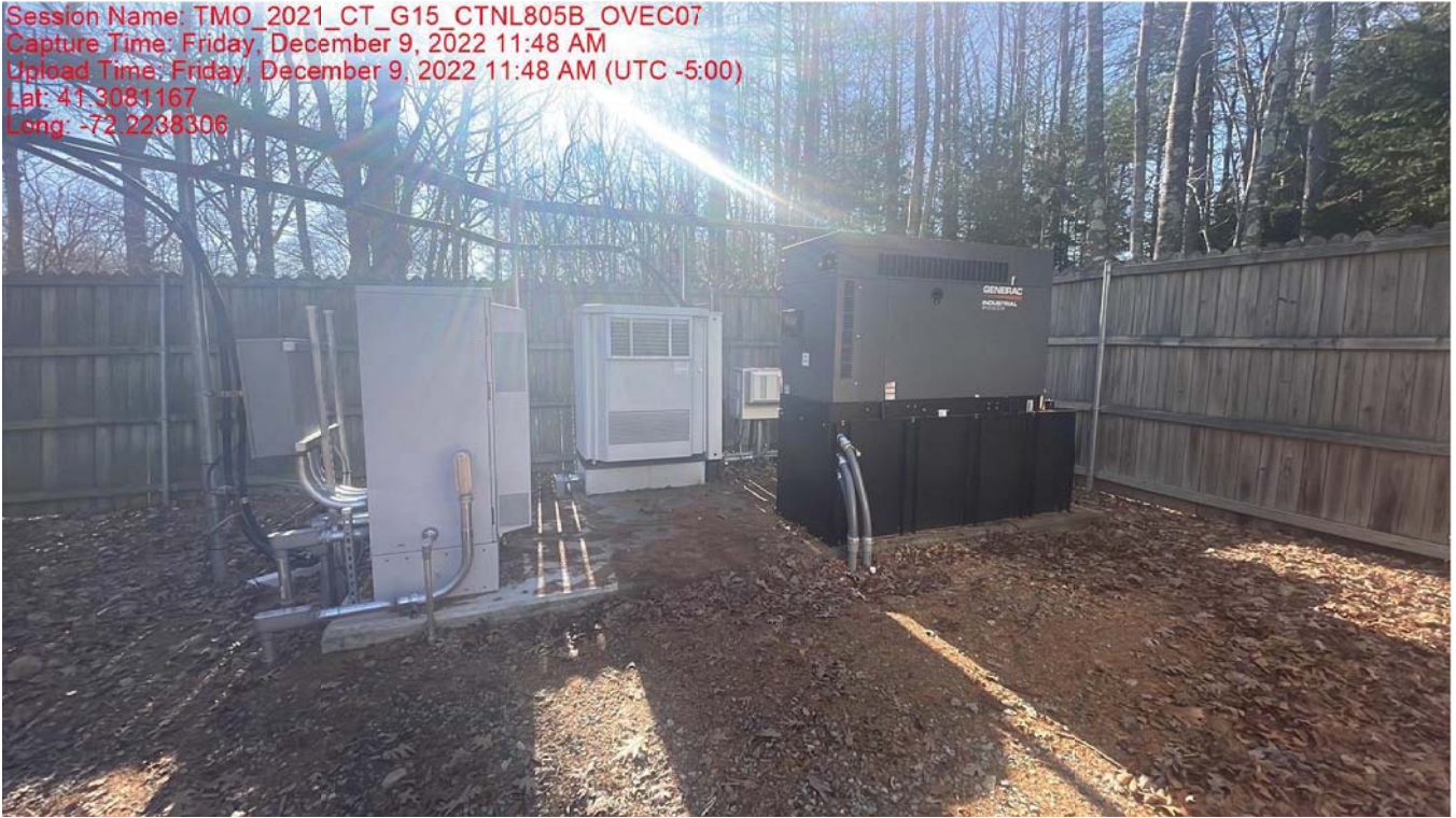
T-Mobile Ground Level Equipment Mounted To Concrete Pad
