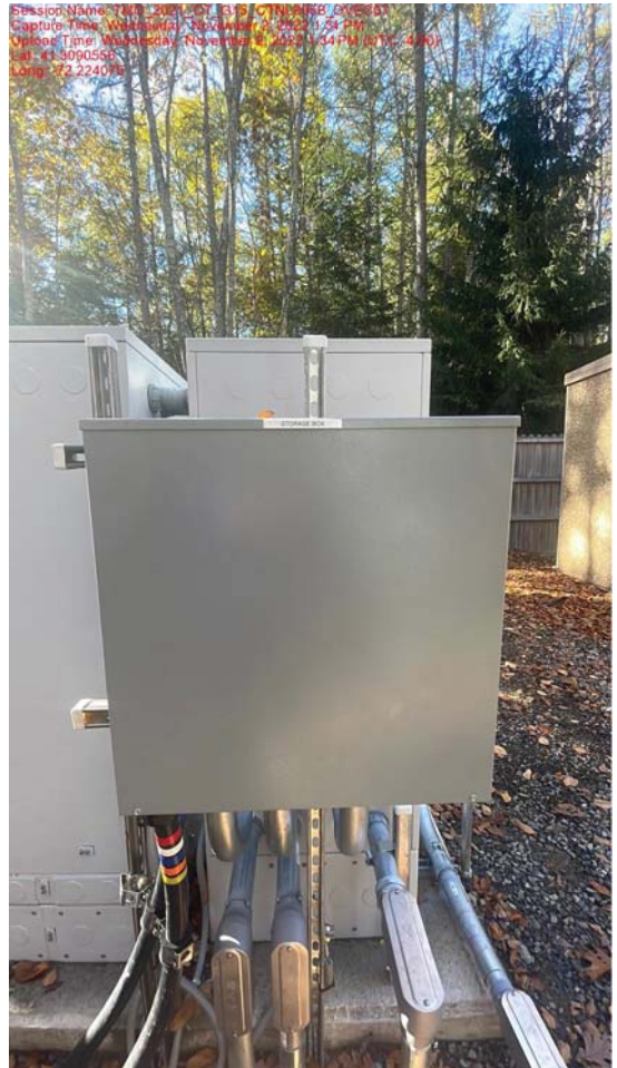
New Slack Box Mounted To New H-Frame
