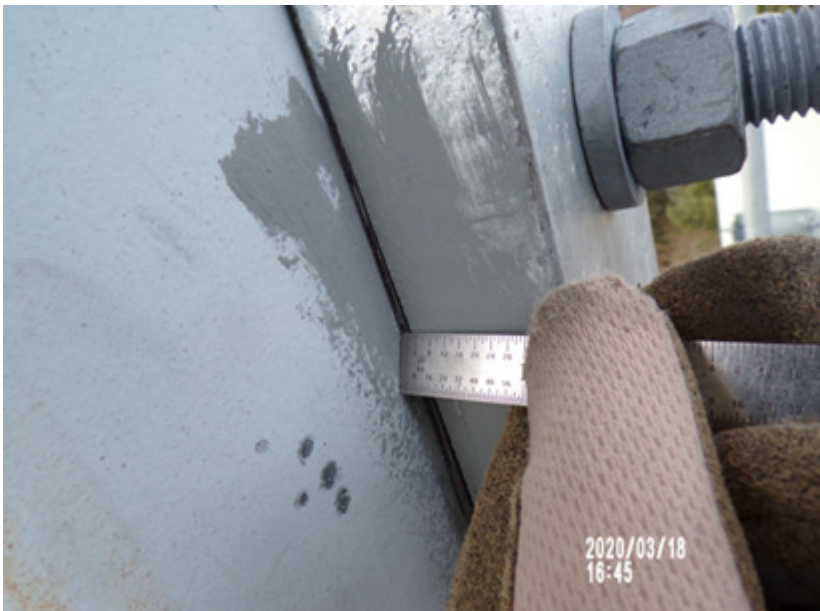
6. Blind bolts have been cut at the flat 11 plate weldment behind the dywidag bar.
