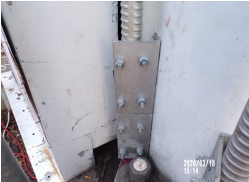
2. Dywidag bars are offset on flats 4 and 10 due to the portholes.
