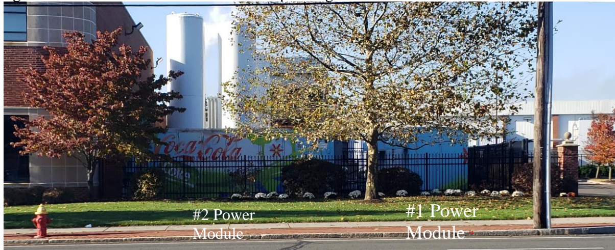
Figure 4. Two Fuel Cell Power Modules Operating at the East Hartford Site
