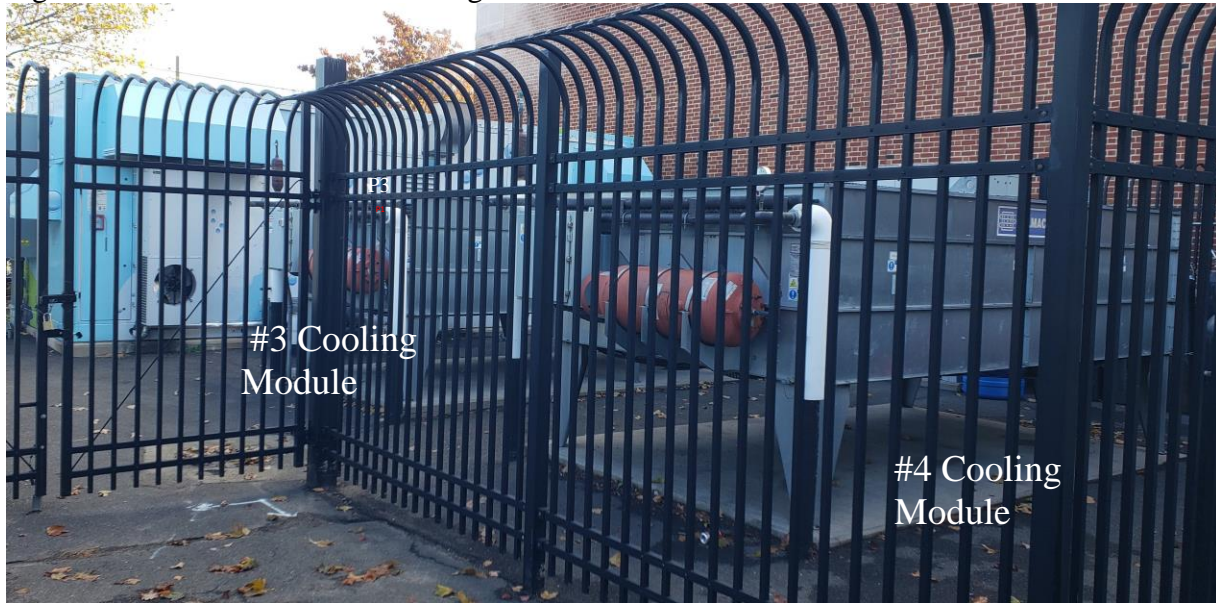
Figure 5. The Two Fuel Cell Cooling Modules at the East Hartford Site
