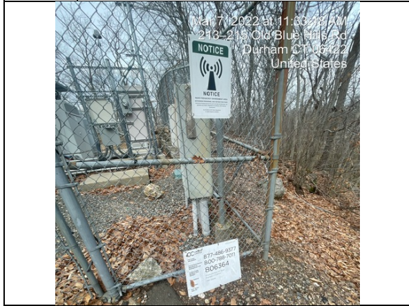
14. Compound Gate Signage
