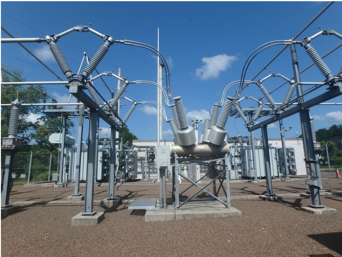
Looking west into existing 115-kV yard at Indian Well Substation Benito Acampora 8/23/18
