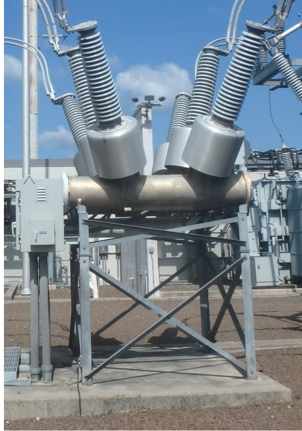
Existing 115-kV Circuit Breaker Benito Acampora 8/23/18
