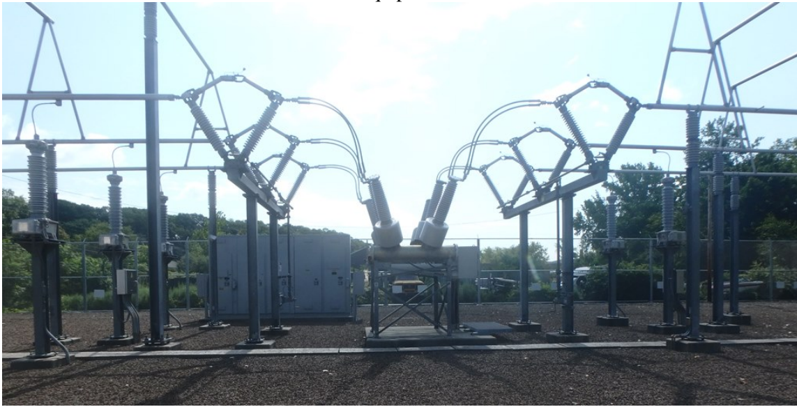
Looking east into existing 115-kV yard at Indian Well Substation Benito Acampora 8/23/18
