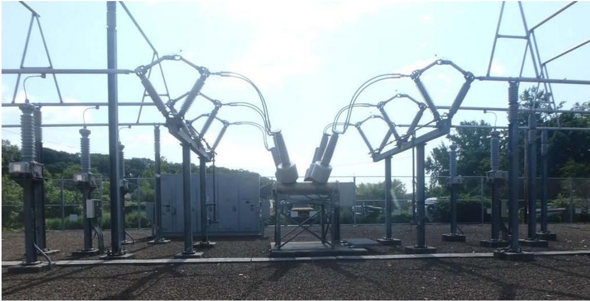
Site and Equipment Looking east into existing 115-kV yard at Indian Well Substation
