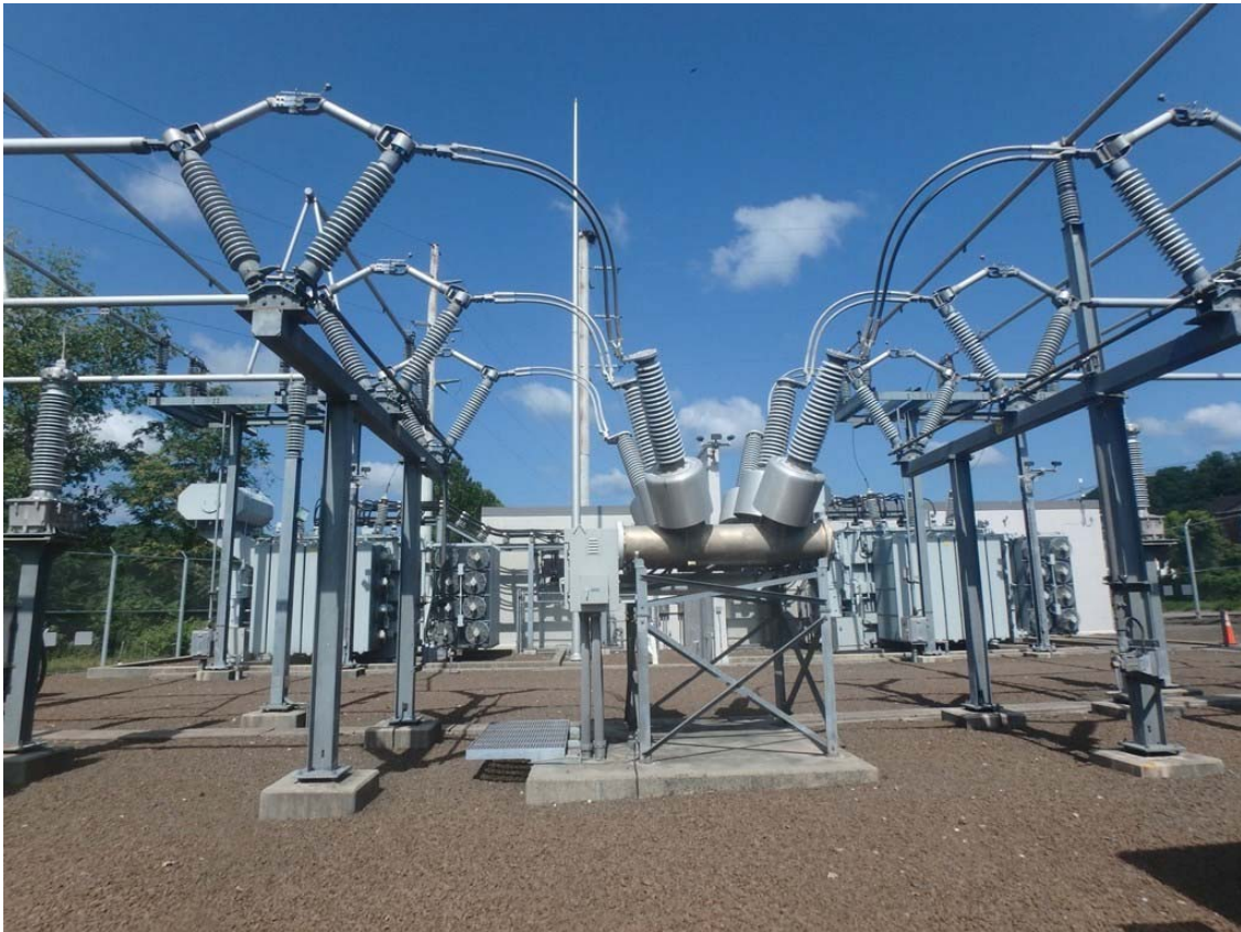
Looking west into existing 115-kV yard at Indian Well Substation
