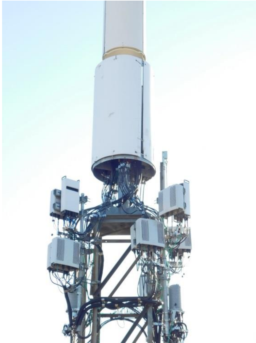
Photo 1: Photo illustrating the Tower with Appurtenances shown.
