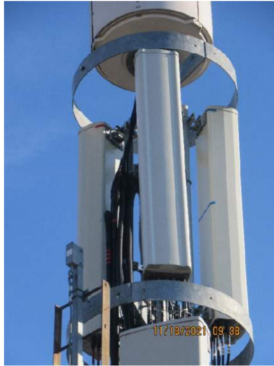
Photo 1: Sample photo illustrating the existing upper section antenna mounts (to be removed and replaced).
