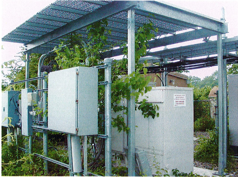
AT&T EQUIPMENT AREA TO BE REMOVED
