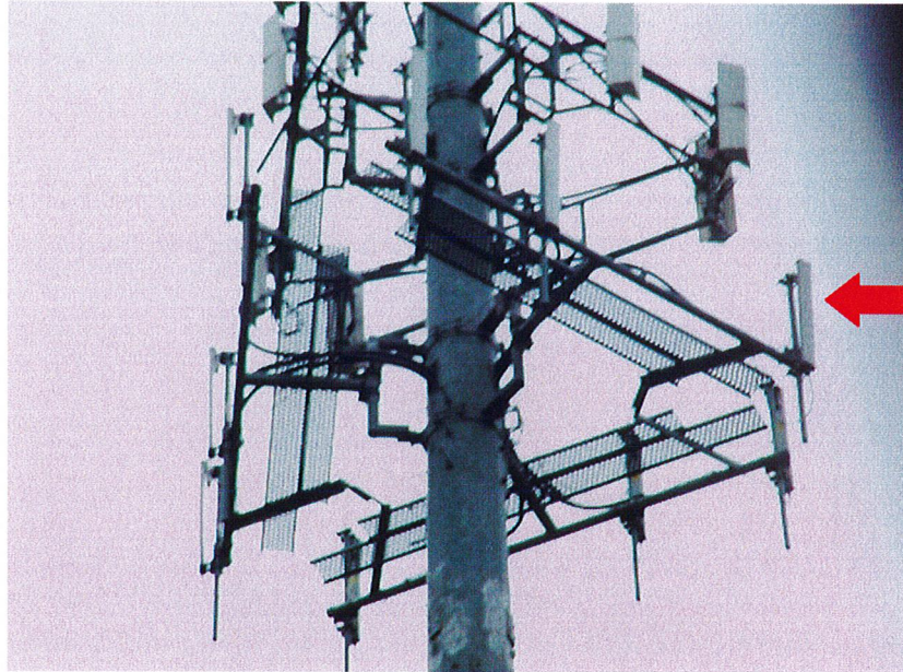
TOWER ARRAY BEFORE
