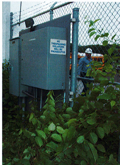
AT&T ELECTRICAL & TELEPHONE EQUIPMENT TO BE REMOVED
