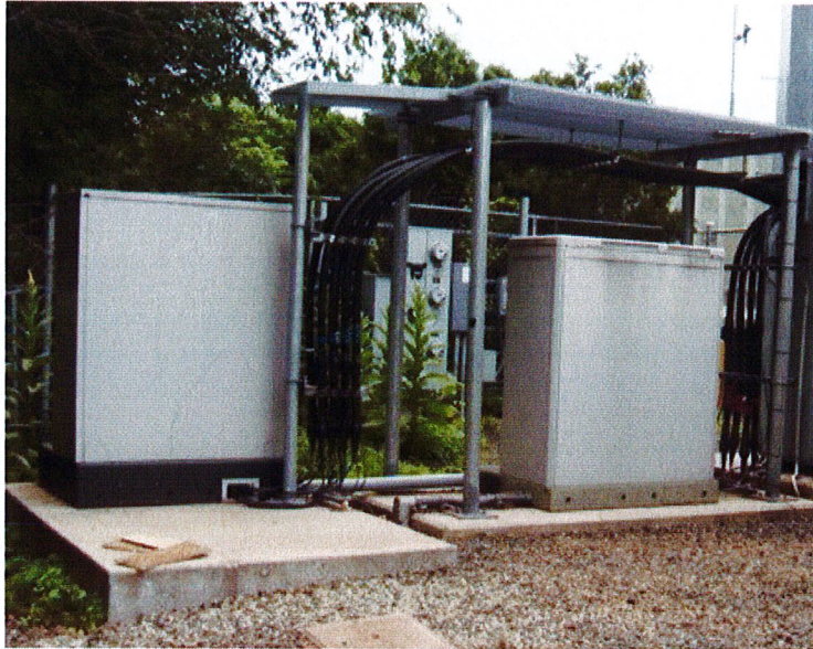
AT&T CABLE ENTRY TO SHELTER AND ASSOCIATED EQUIPMENT
