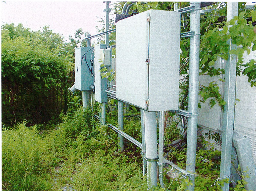
AT&T ELECTRICAL & TELEPHONE EQUIPMENT TO BE REMOVED
