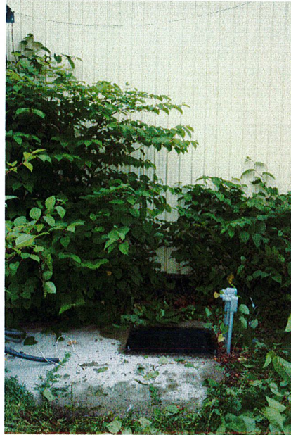
AT&T PAD & ASSOCIATED EQUIPMENT TO BE REMOVED
