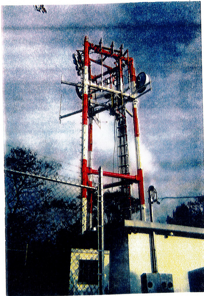
Photo #2. 65' Steel Radio Tower
