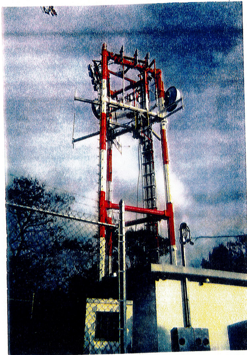
Photo #2. 65' Steel Radio Tower
