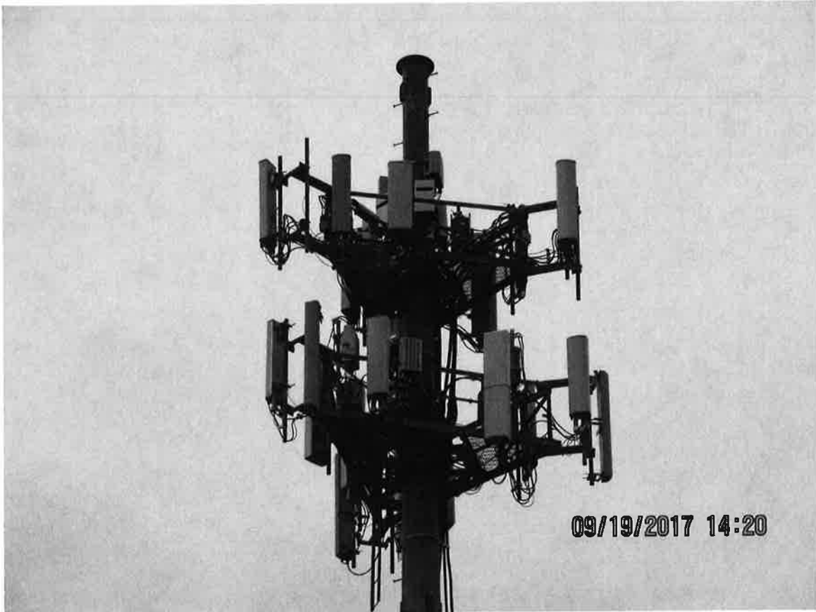
Photo 1: Photo illustrating the monopole with Appurtenances shown.
