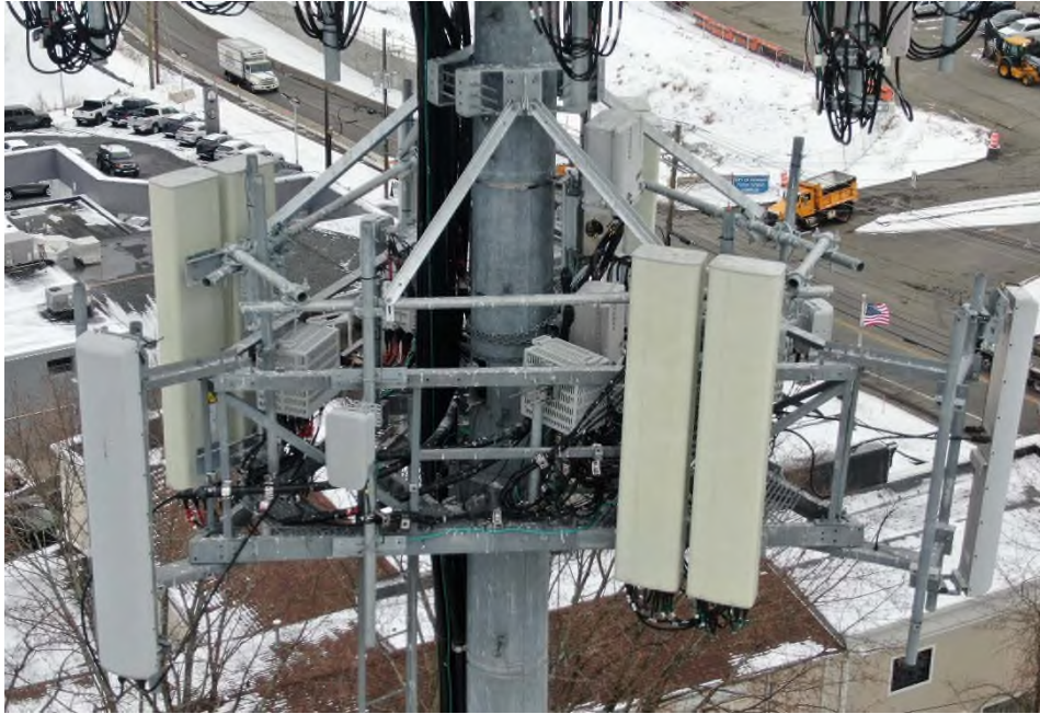
Photo 1: Photo illustrating the monopole with Appurtenances shown.
